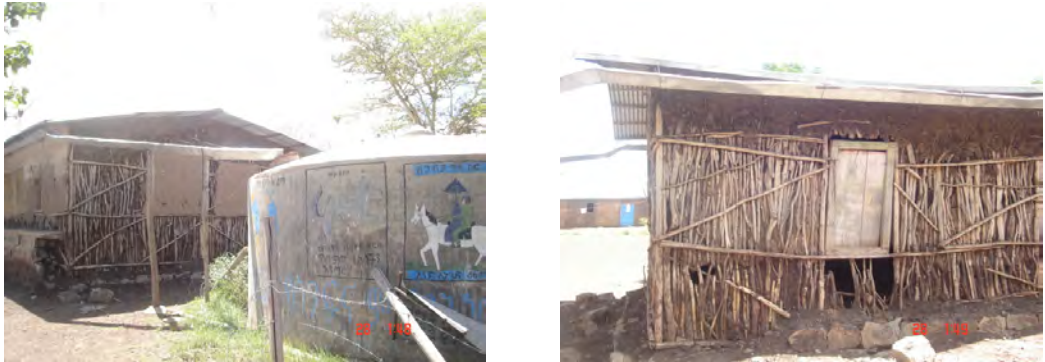
Figure 5-2: 40 m 3 Ferro cement reservoir fixed with a nearly damaged school block (Chele School)
