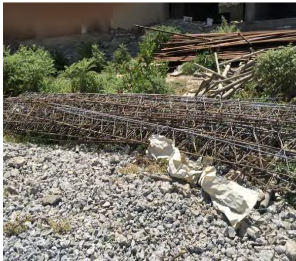
→ Rebar prepared for precast beams just laid exposed on site wasted
