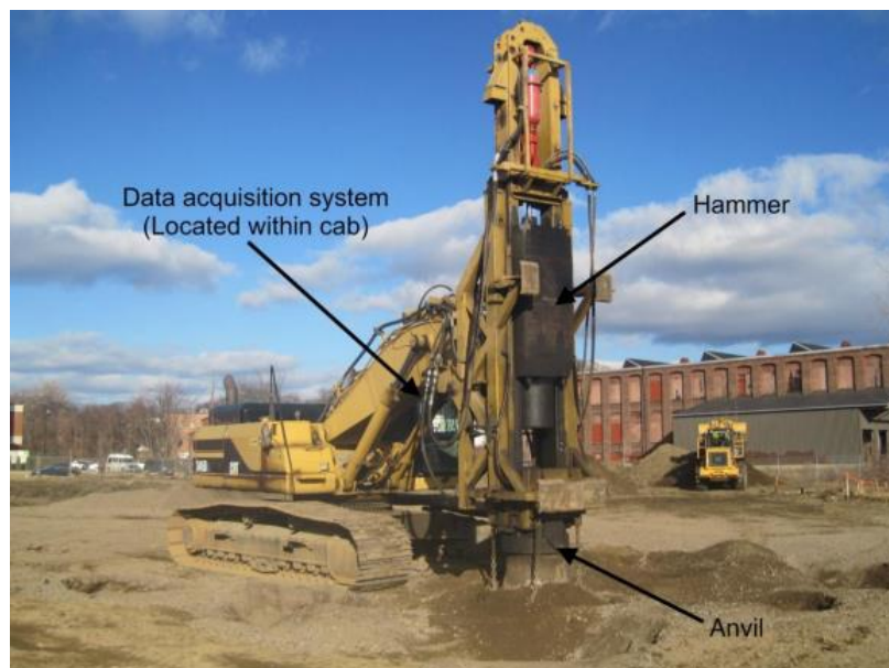
Figure 7: A Typical RIC Unit (Source: P.J. Becker [2011])
