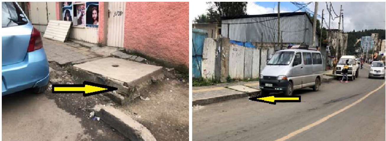
Figure 4- 6: Existing blocked drainage manholes
