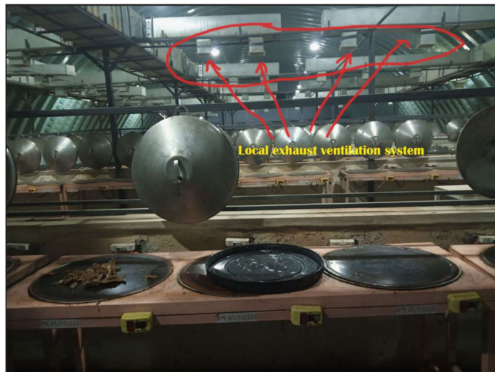
Figure 14: shows the ventilation system of Injera Baking Center.
