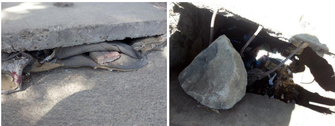
Figure 5.3: Blocked and damaged manhole (Source: Temanja station)
