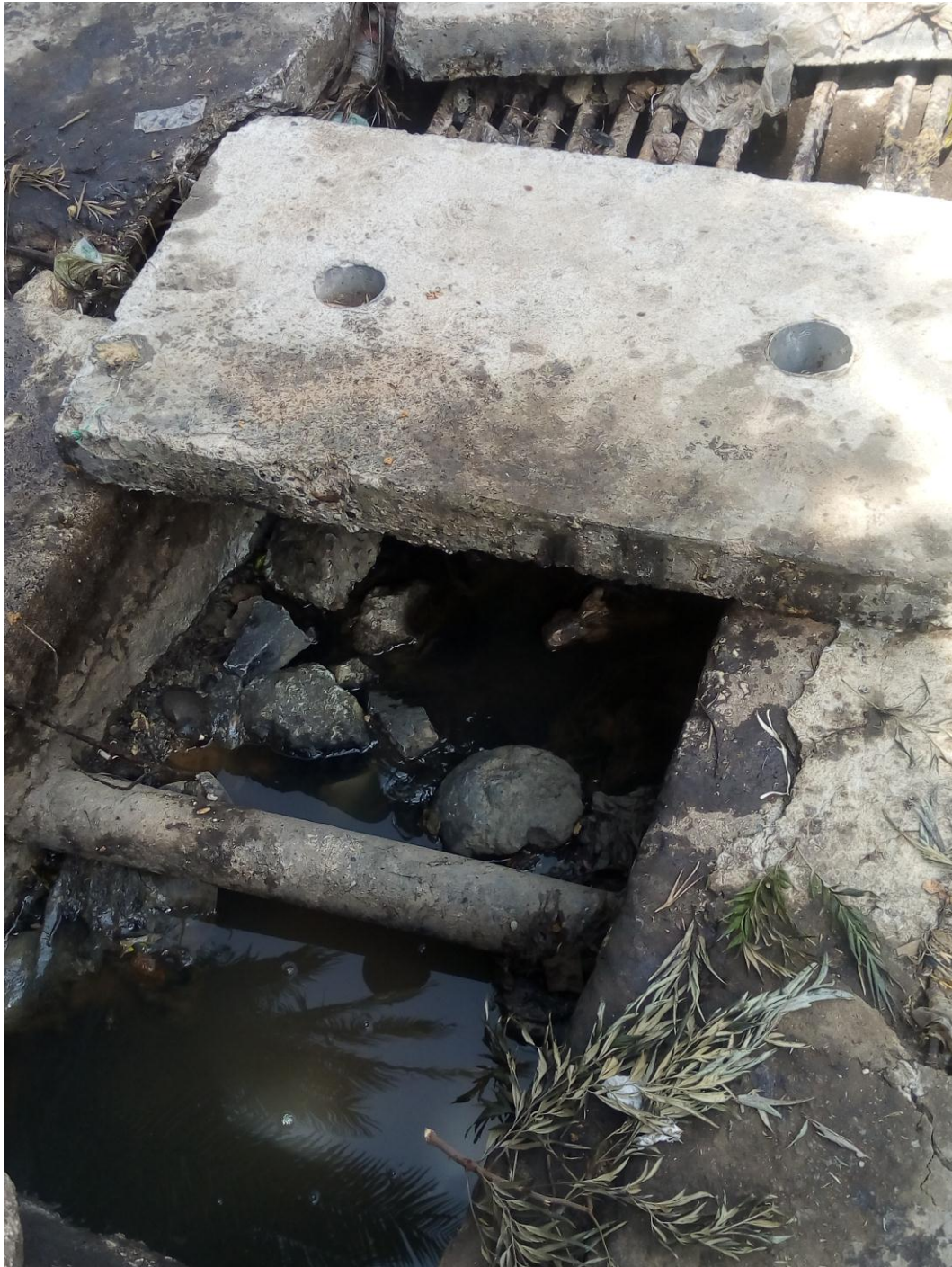
Figure 5.19: Drainage point at total petrol station (Source: Temanja station)
