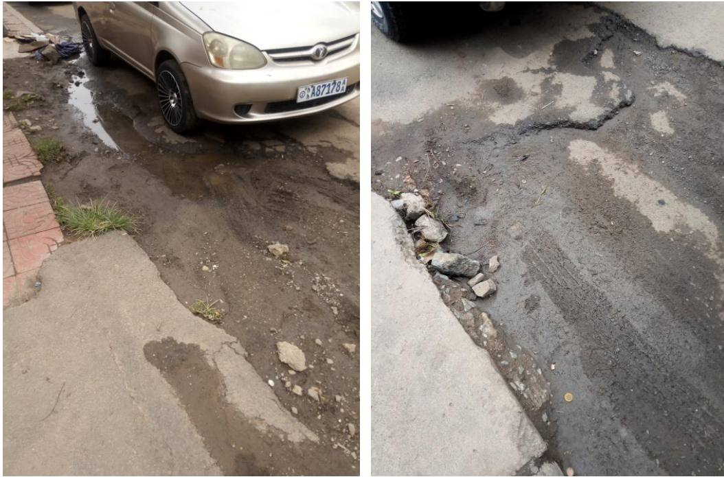
Figure 5.12: Presence of silt on the roadway
