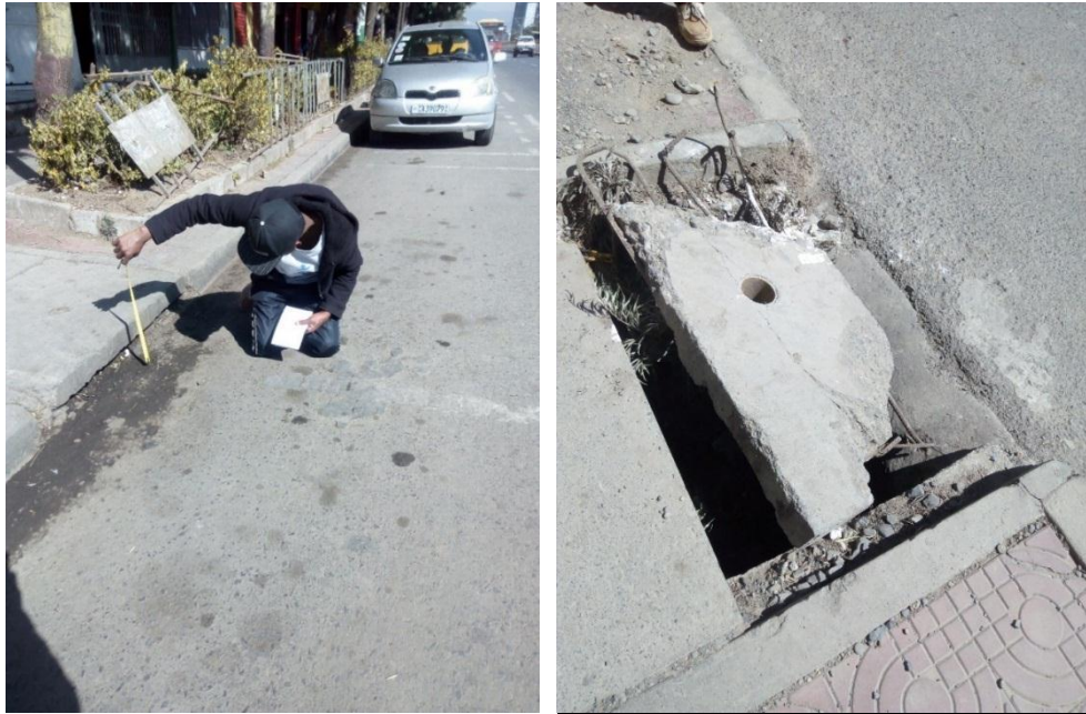
Figure 5.4: Measurement of entry width and dismantled cover of the manhole (Source: Richie station)
