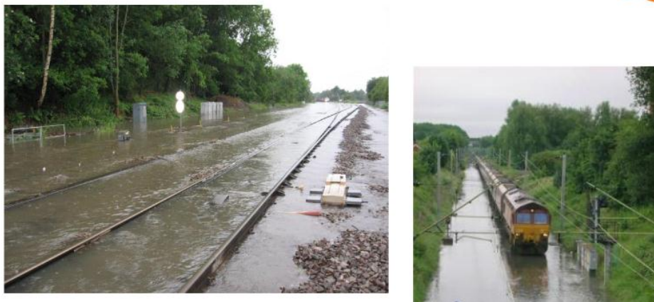
Figure 2.6: Flooded railway track
