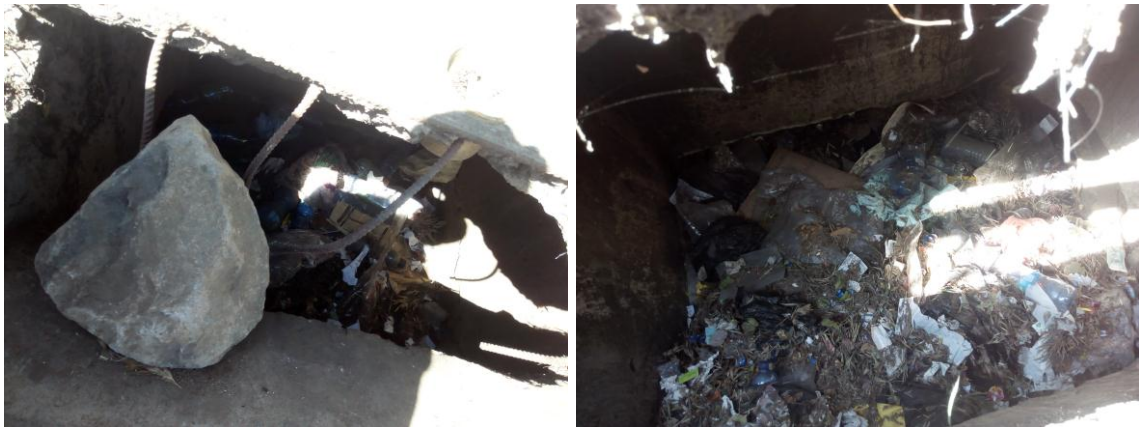
Figure 3.12: Rubbish within manholes
