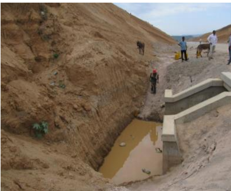
Fig 4.5 buried culvert invert level deep into the ground compared to the surrounding ground levels.
