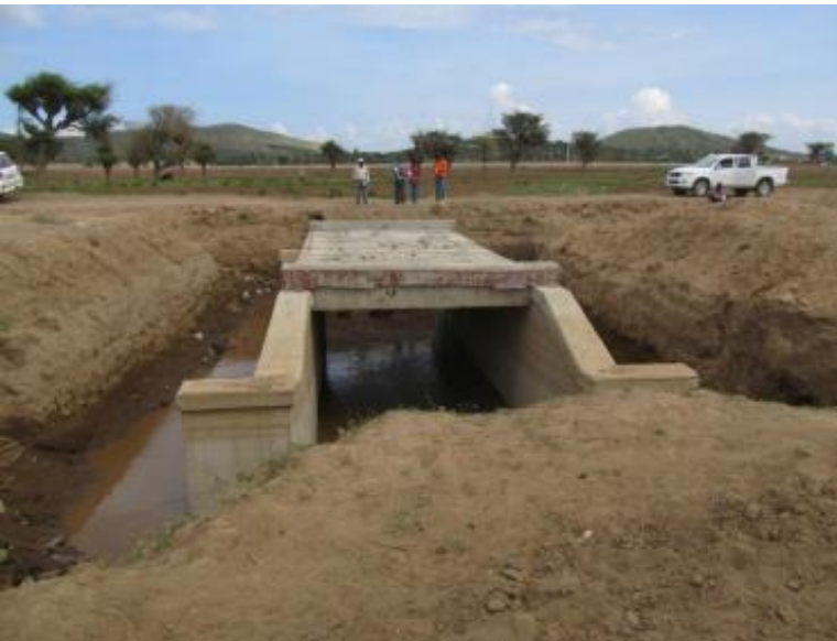
Fig 4.4 incorrectly oriented Culvert Structure
