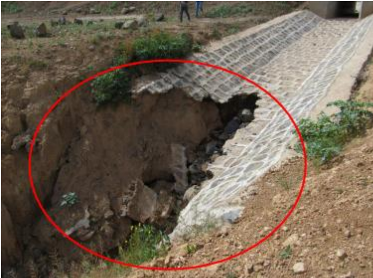
Fig 4.3 Damaged outlet structure
