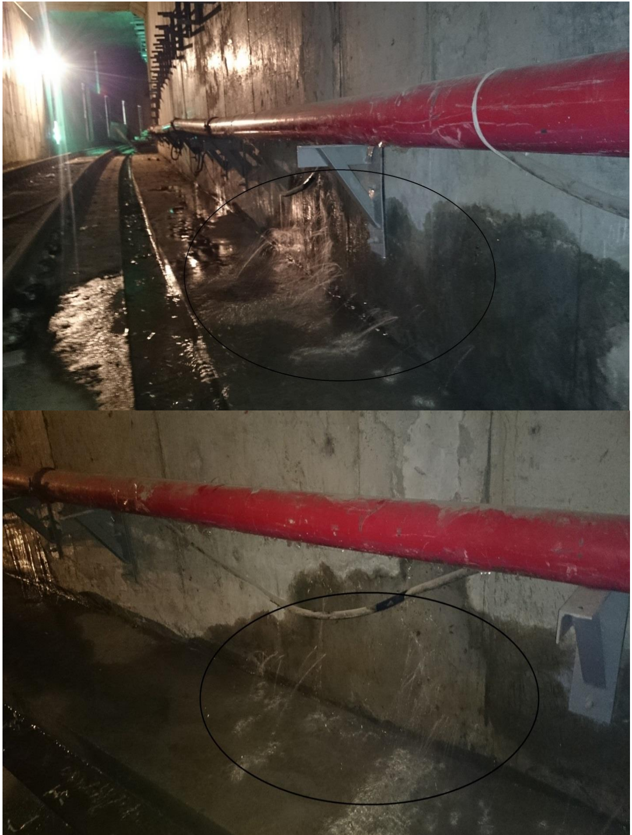
Fig.4.2 Water Flow inside the Tunnel of Addis Ababa LRT before remedial measure taken
