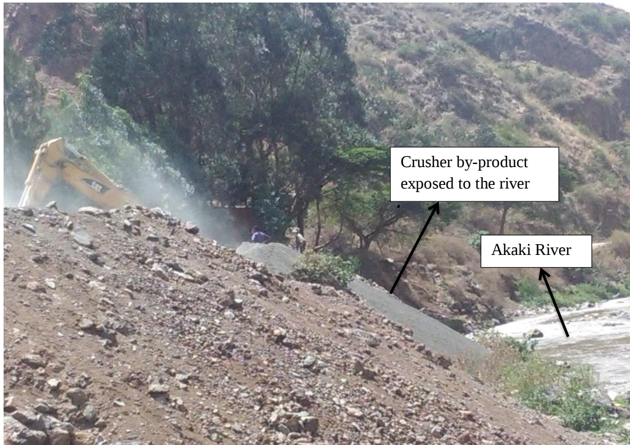
Figure 6-2 Dumping of crusher by-product to adjoining river (aggregate production sites around Akaki River)
