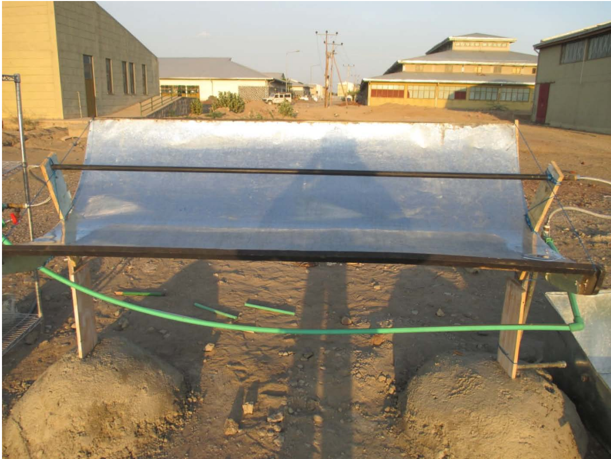
Fig 3.4: Installed Parabolic Solar Concentrator
