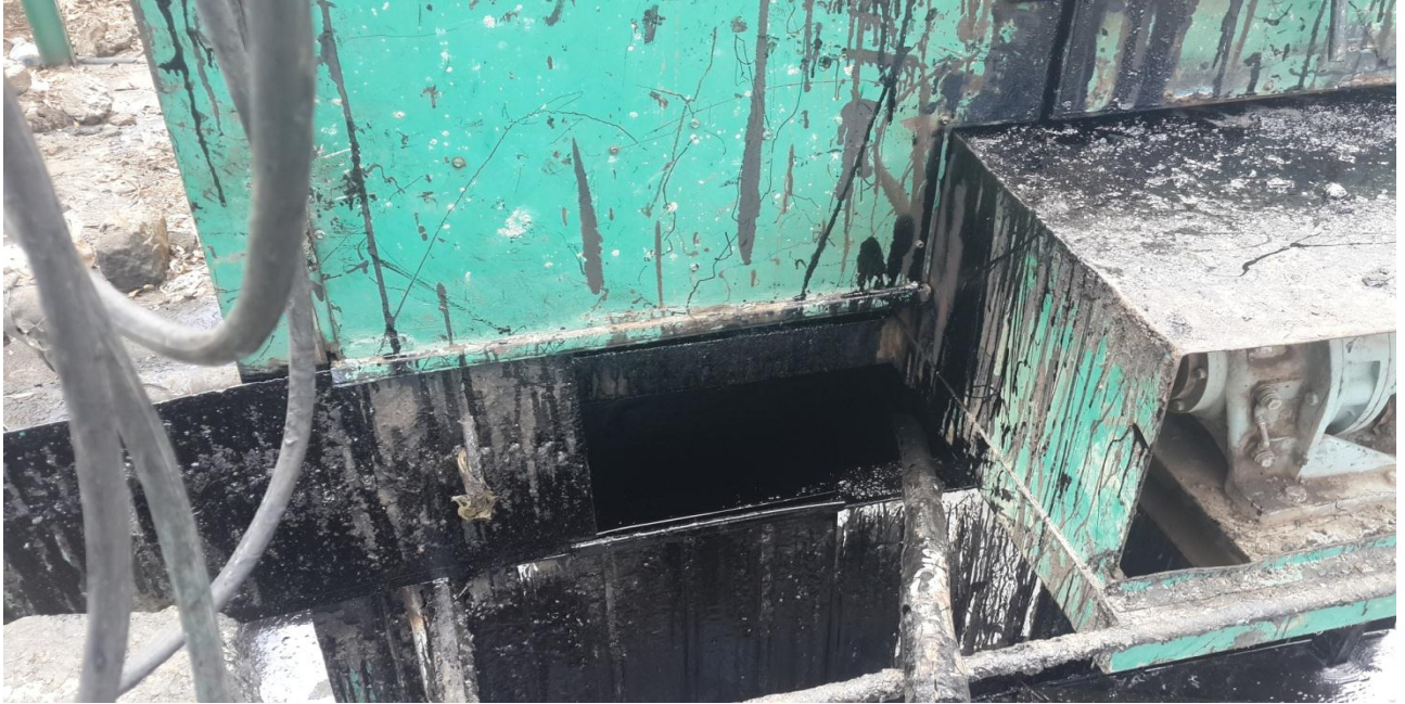
Figure 11 Akaki Asphalt Storage Tank
