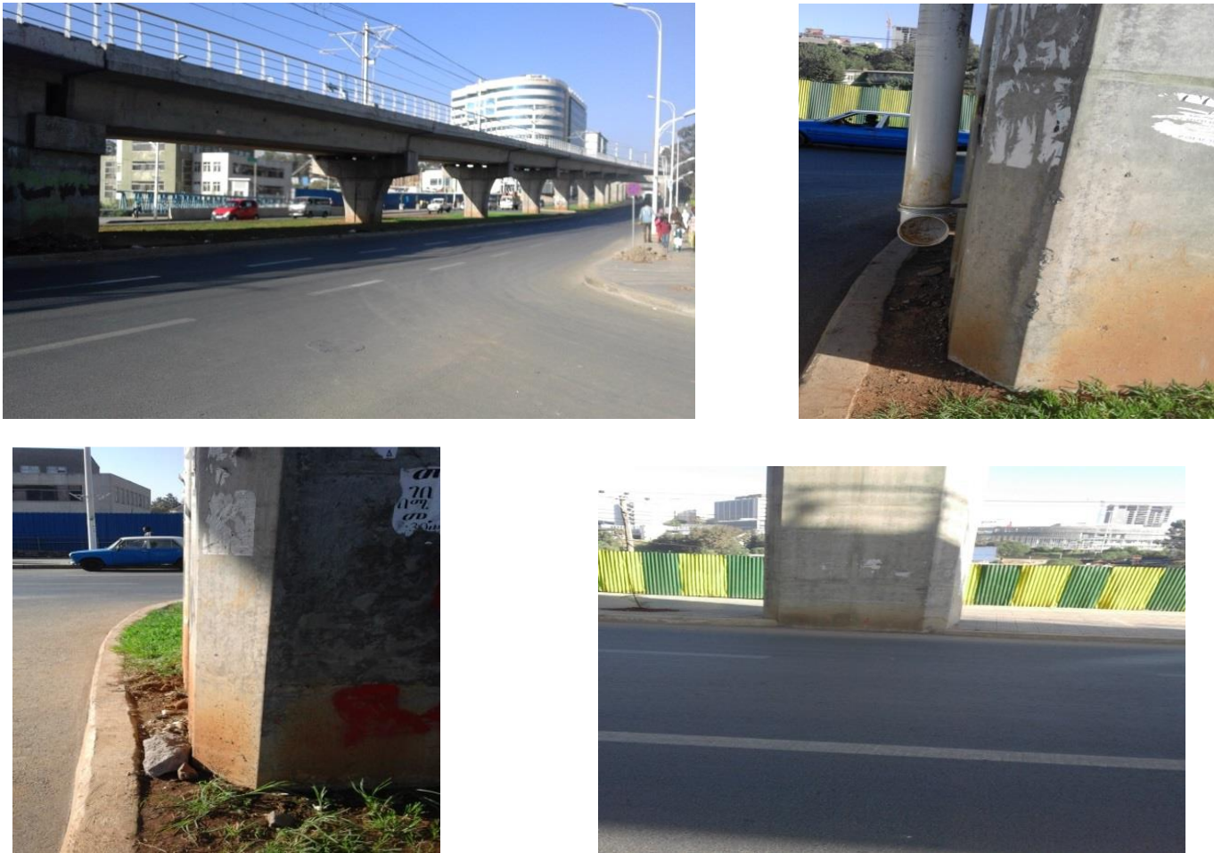
Figure 3-15 Photographs shows exposed for vehicle collusion on Railway Bridge piers around Bambis area
