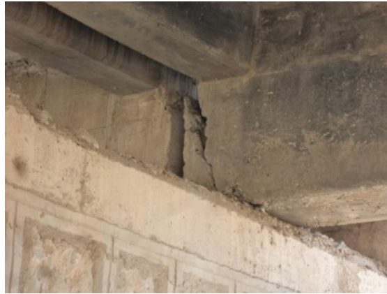
Figure 3-12 Shear crack, void and spalling on C100-1-047 River Bridge
