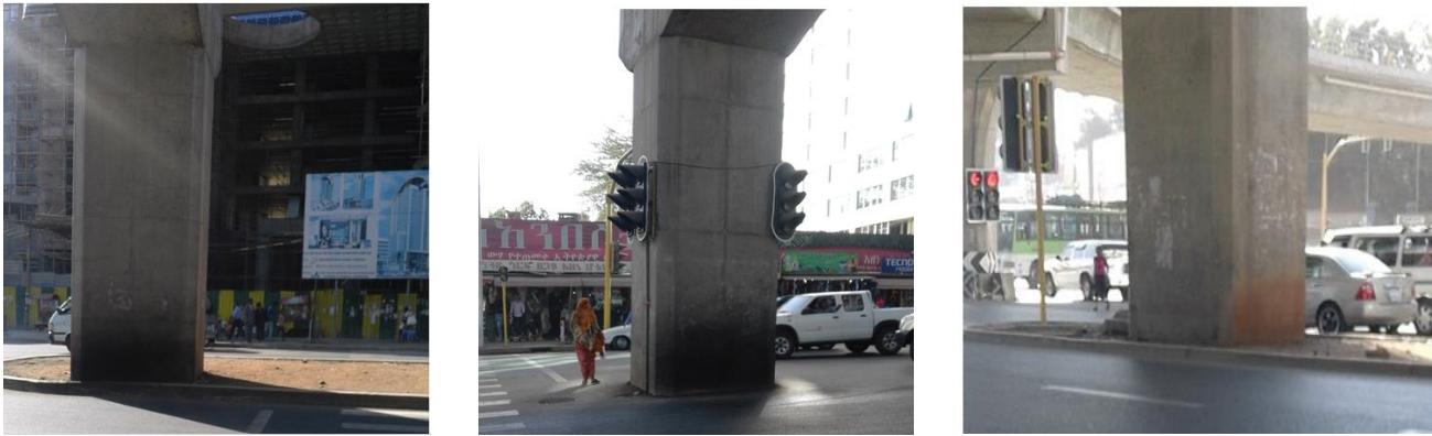
Figure 3-16 Photographs shows exposed for vehicle collusion on Railway Bridge piers around stadium area
