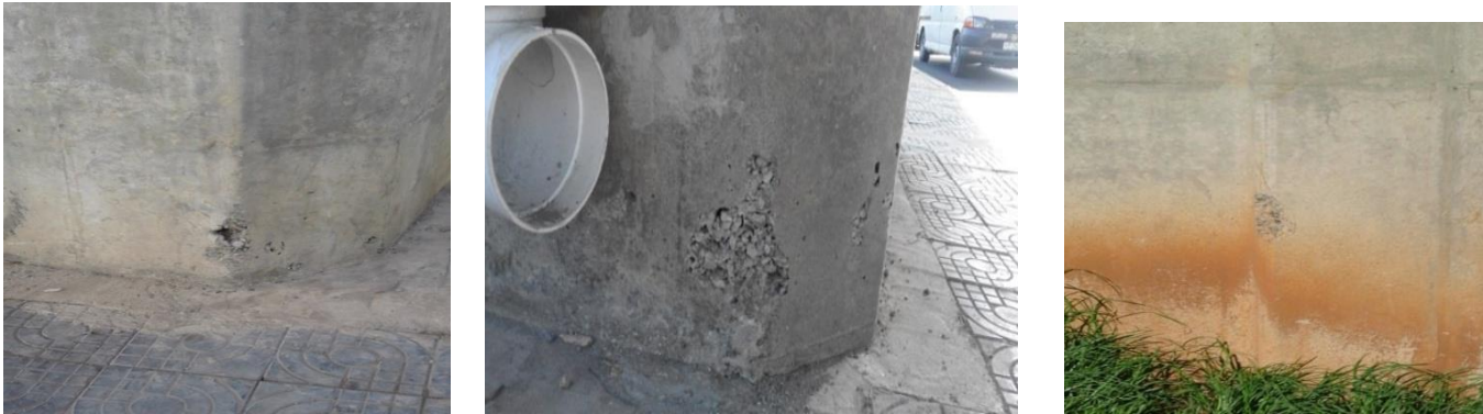
Figure 3-14: Photographs shows spalling on Railway Bridge Piers around Bambis area
