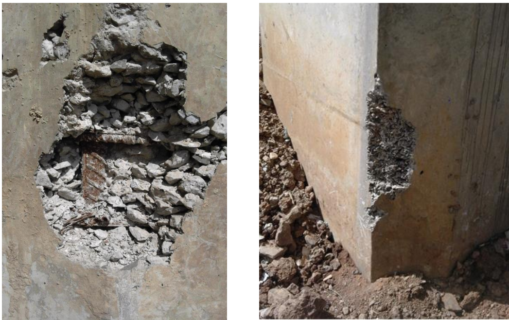
Figure 3-17: Photographs shows rebar exposure & spalling on Railway Bridge piers around Firdbet area
