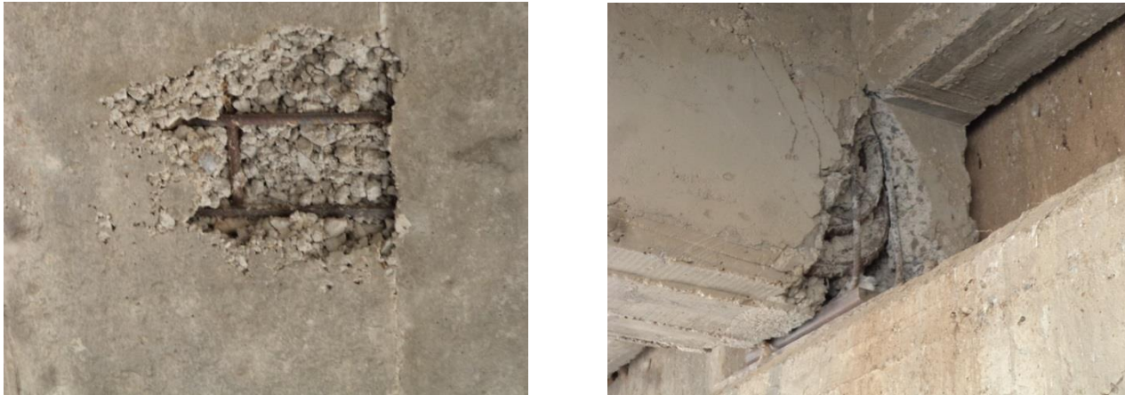
Figure 3-8 Shear crack, corrosion, spalling, bearing & bearing plate damage on C100-1-018
