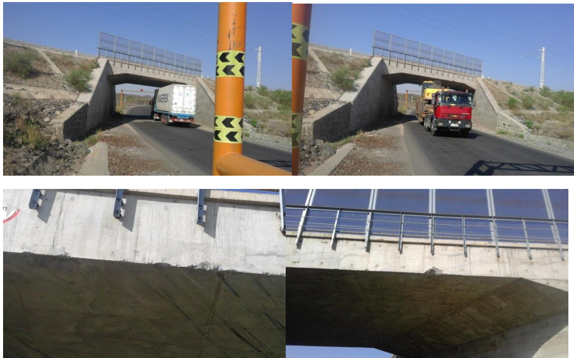
Figure 3-1 Potential damage on overpass Railway Bridge by under passing vehicular impact, around Welenchiti
