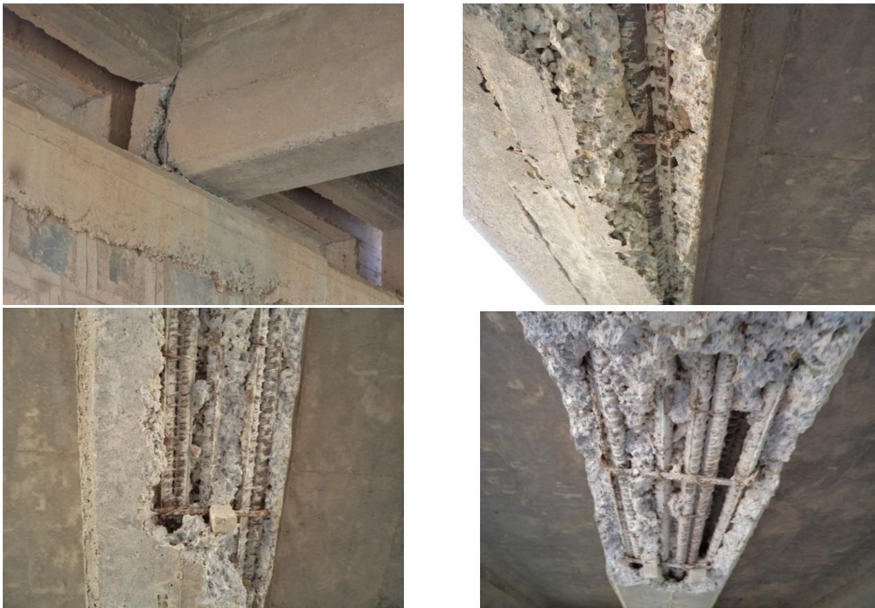
Figure 3-9: Corrosion, shear crack, spalling damage on C100-1-019 (Harmukali) River Bridge
