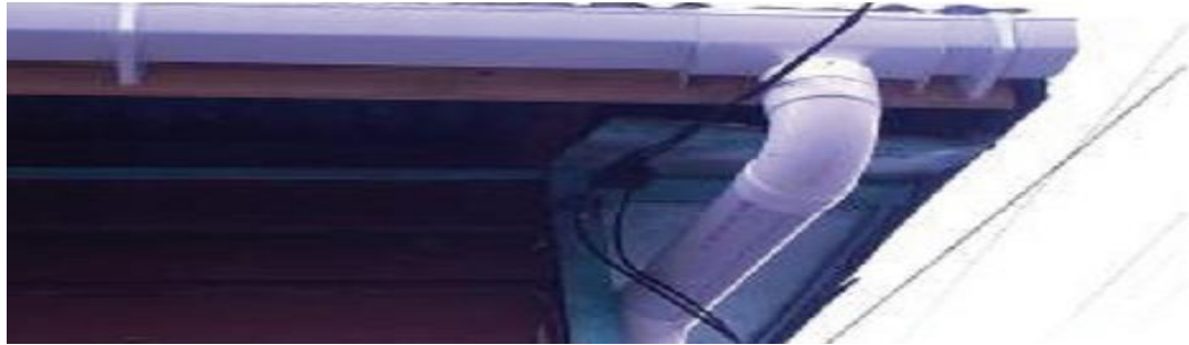
Figure 38 Gutter and downpipes used for RWH system, 2015
