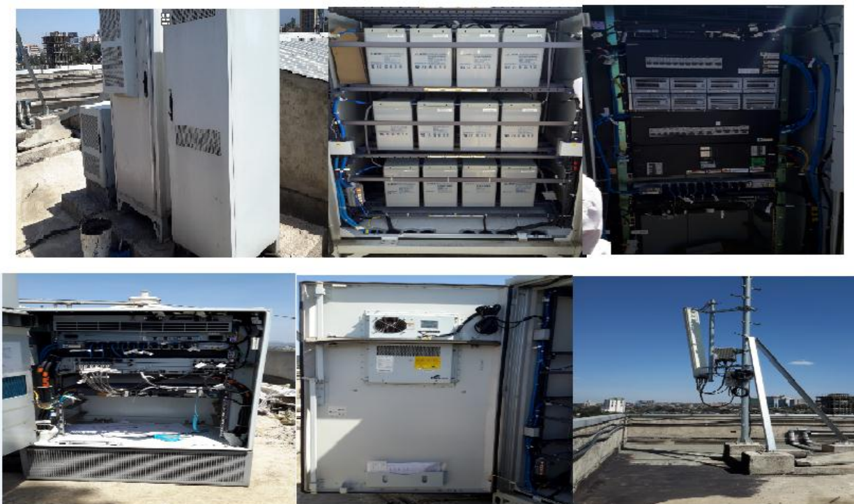
Figure 3.2 outdoor tower and equipment a camera picture (Sarem Building AA, January 2016)
