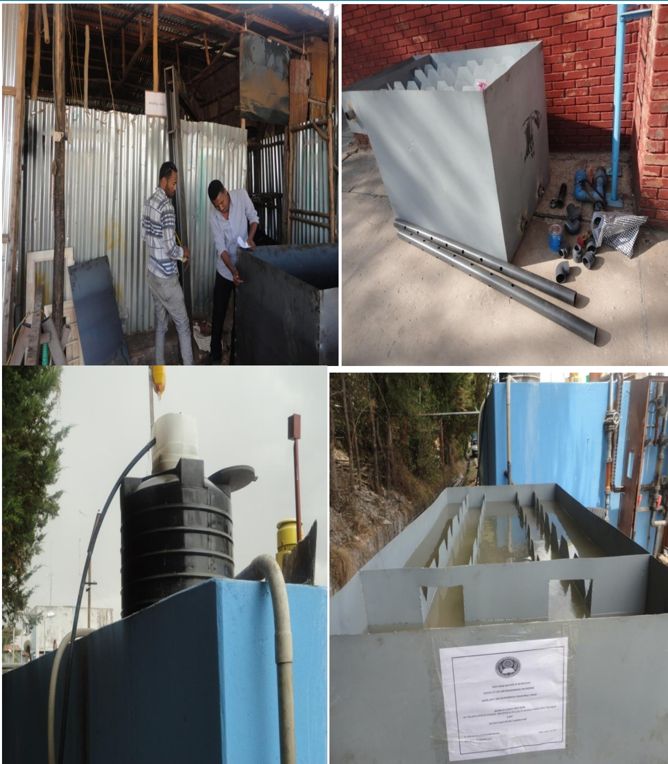
Figure 3-8: photos of the constructed and installed systems of the pilot plant.
