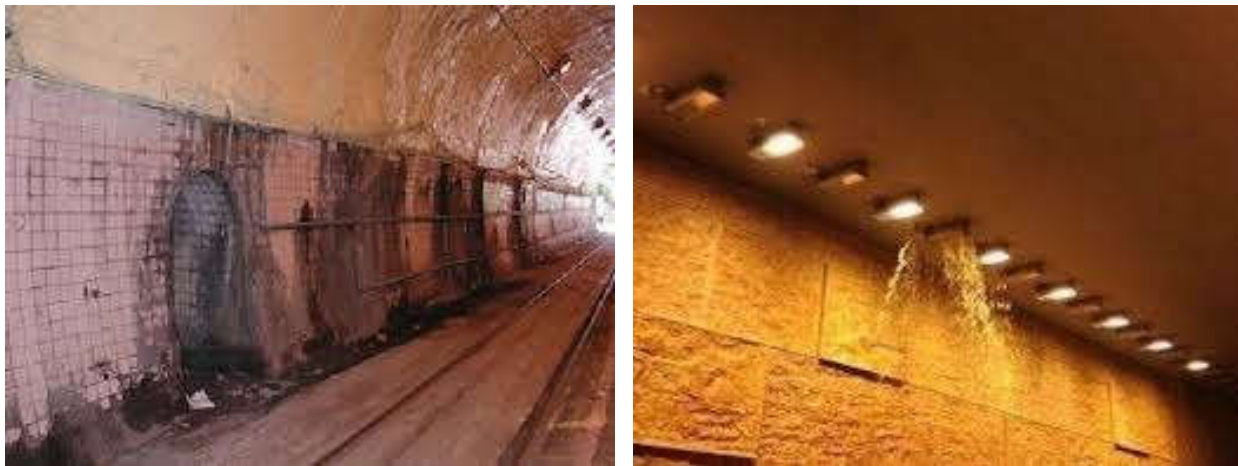
Figure 8 Leakages in tunnels
