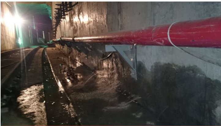
Figure 6 Side wall leakage
