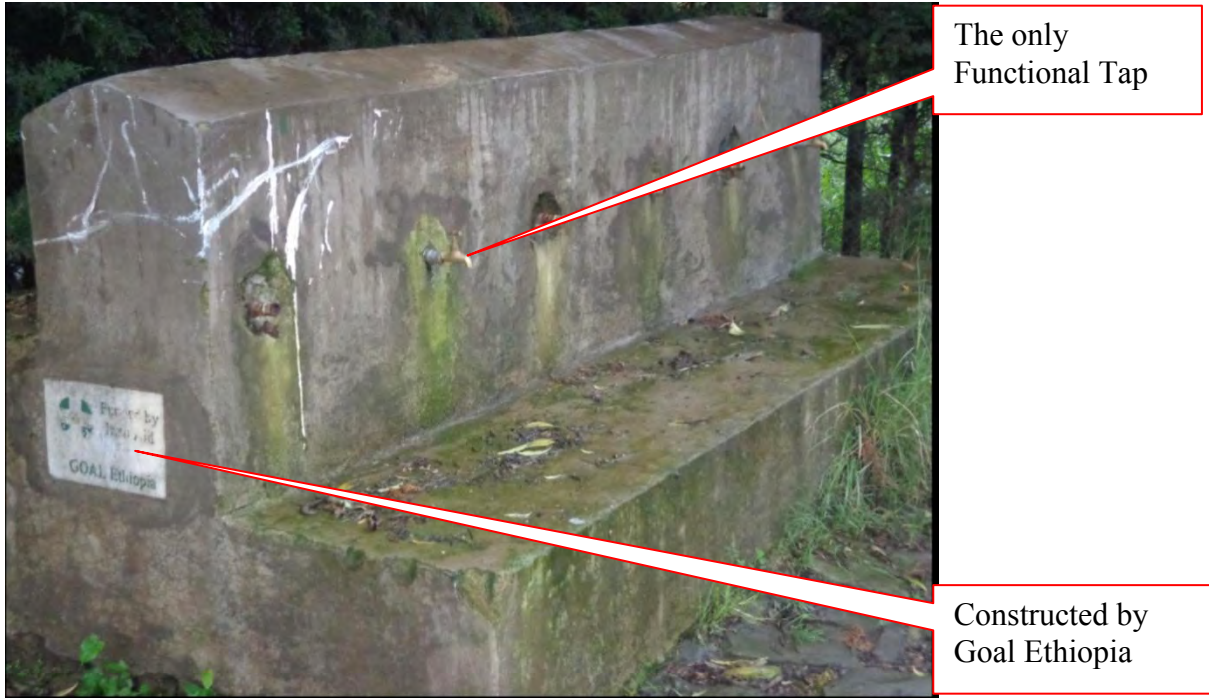
Photo 4.1 Only One Functional Tap Piped Municipal Water Supply (Source: Personal field survey, 2016)
