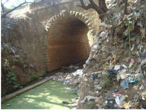
Plate 6.3. Waste disposal on river banks
