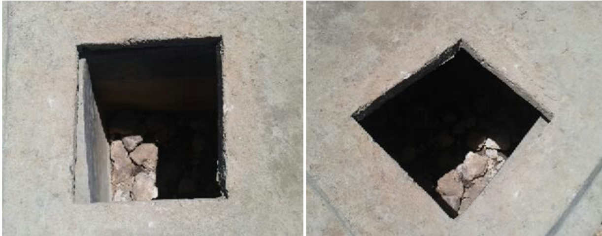
Figure 4.29 Spring box structure with no water
