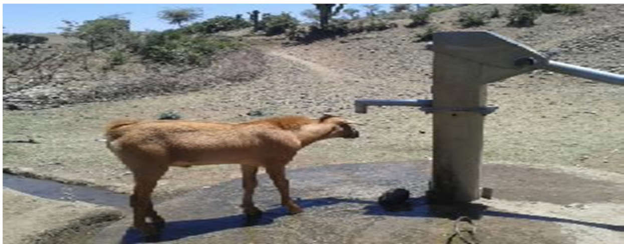
Figure 4.35: HDW with no fence exposed to animals and children's
