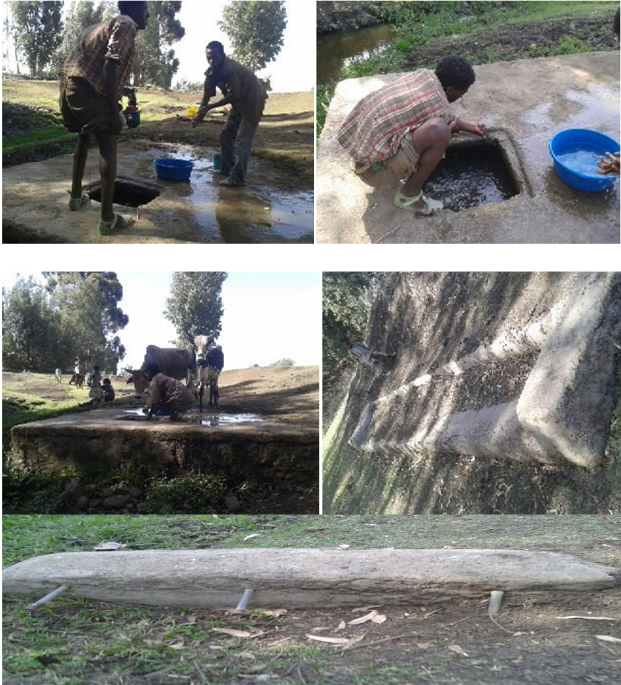
Figure 4.31: Failed spring component due to poor site selection
