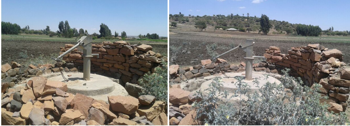
Figure 4.25 Dry HDW with damaged fence
