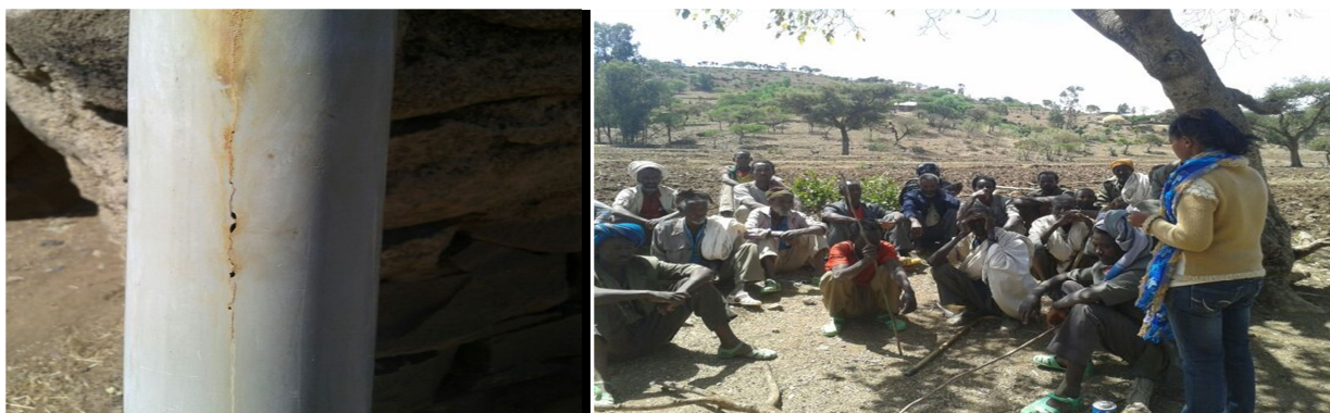
Figure 4.34 Cracked PVC and discussion with water point users
