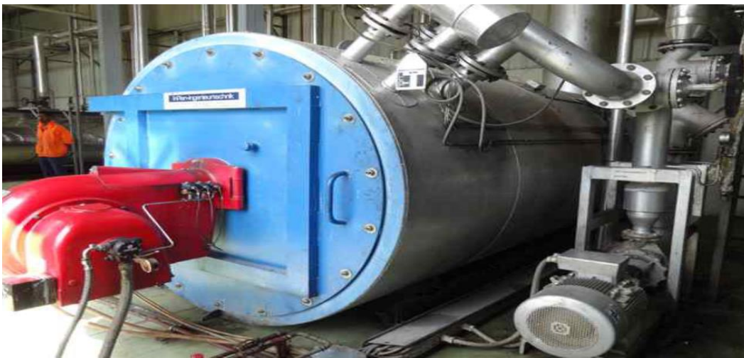
Figure 3-19: Thermo boiler installation view
