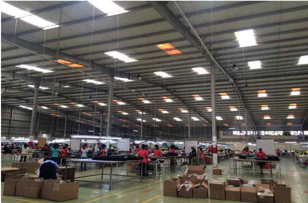
Figure 4-9: Lighting installation of garment department
