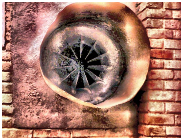
Fig.25 External view of the fan for cooling the electric motor.
