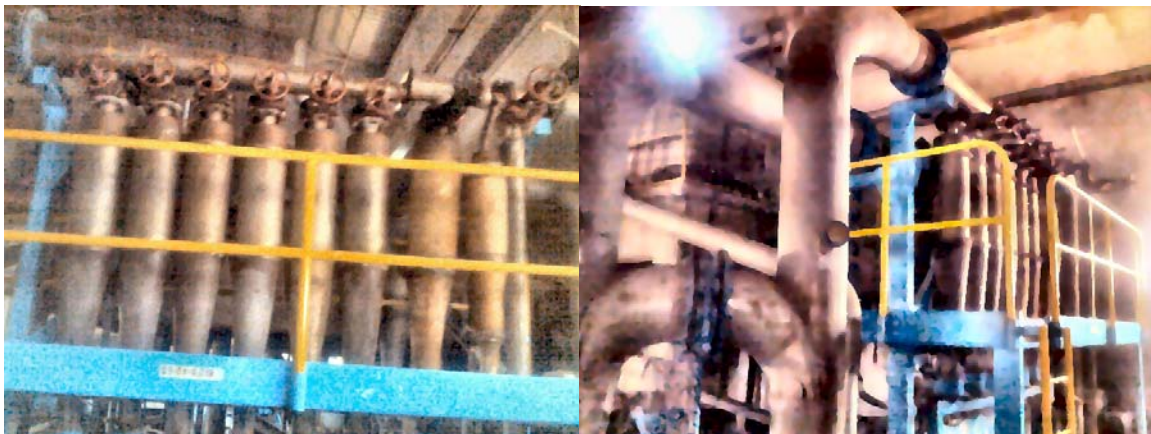
Fig.11 Cyclonic separator in the factory
