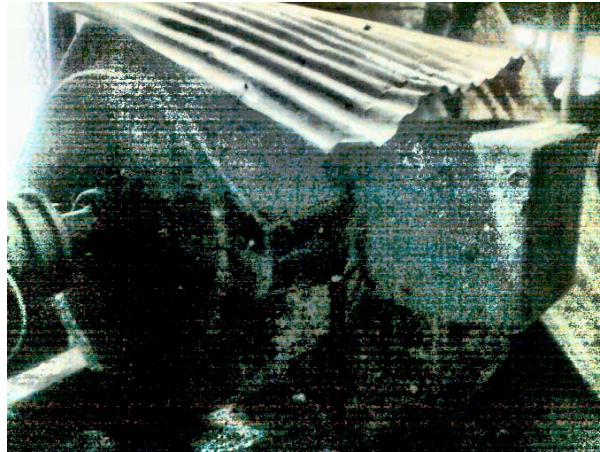
Fig.24 Electric motor driving the line shaft.
