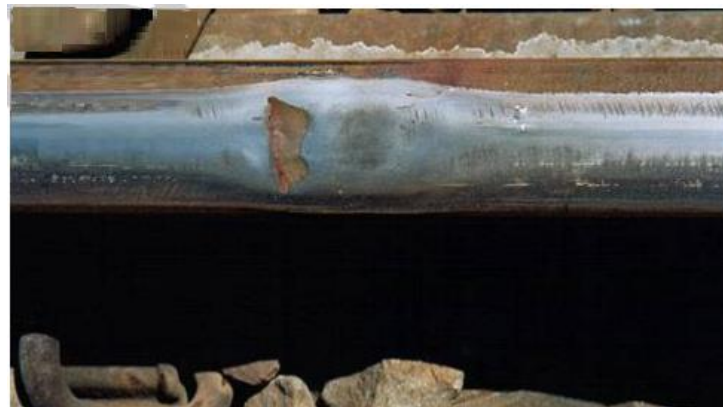
Figure 2.16 Rail Crown Squats (U.S. Dept. of Transportation, 1984)
