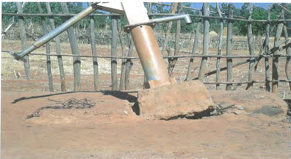
Figure4.4: Nonfunctional HDW in Assero Gote of Yenscha Kebele , Poor Construction quality.
