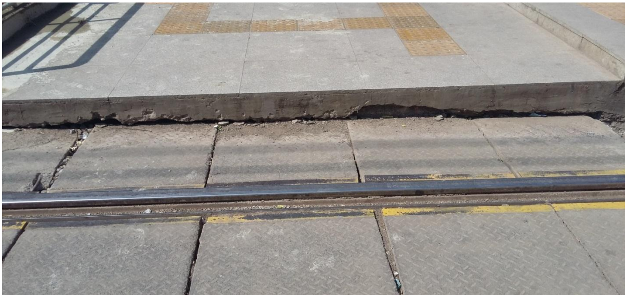
Figure 4.1 Wheelchair users difficulties to cross through the LRT line
