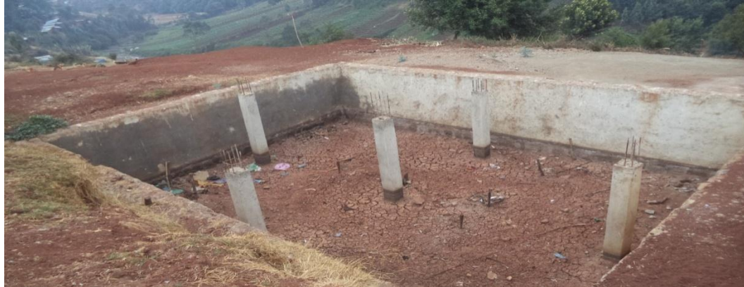
Figure 4.3: Municipality's abattoir treatment plant
