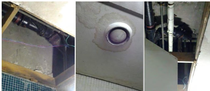
Figure 3- 36 Microbial growth and dampness in the toilet
