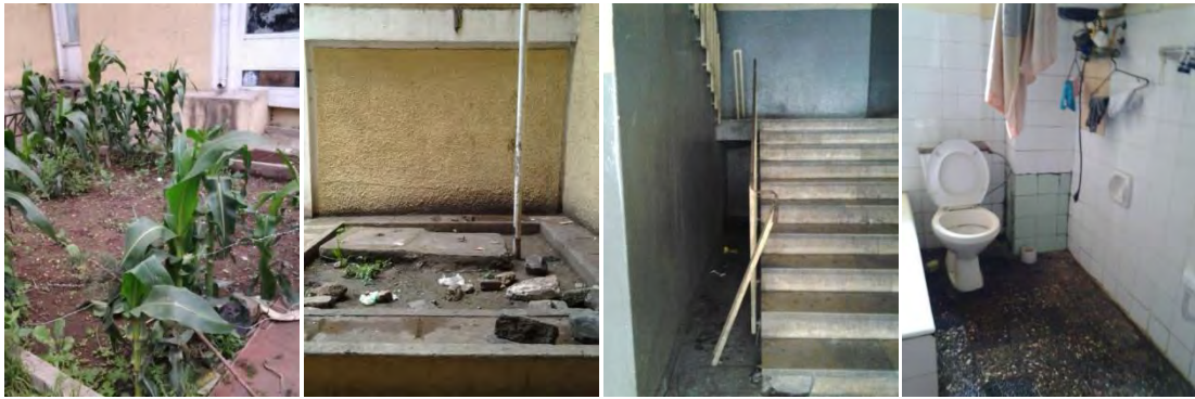
Figure 3- 59 Unmanaged green infrastructure microbial growth and dampness within the apartment
