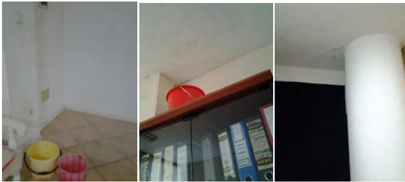
Figure 3- 24 Leakage on roofs and terrace
