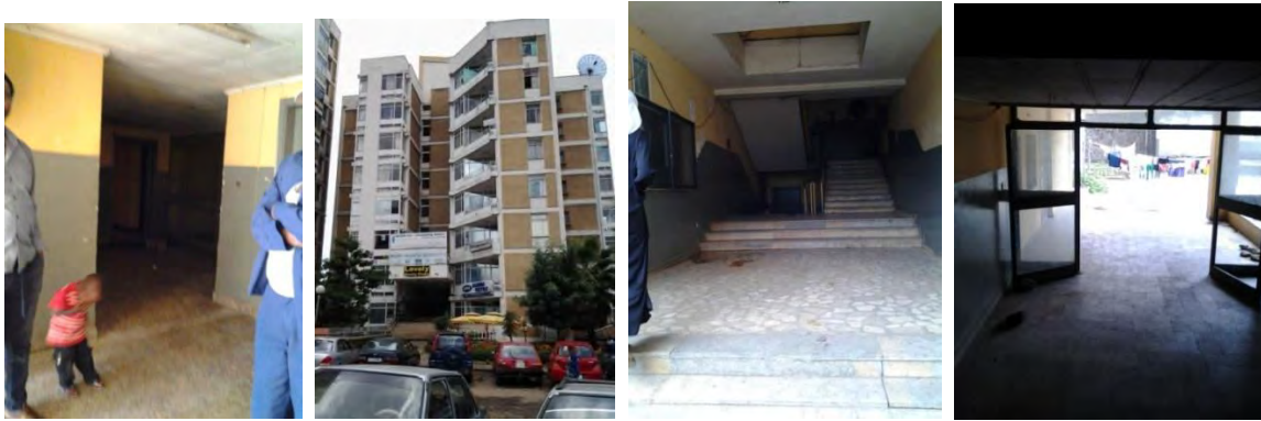
Figure 3- 58 Some worn out facilities in the apartment and the entrance of the apartment
