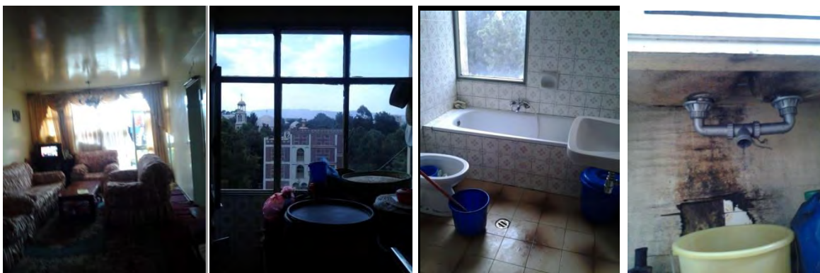
Figure 3- 73 Windows of the apartment and floor drainage causing dampness and kitchen fixture leakage causing damage
