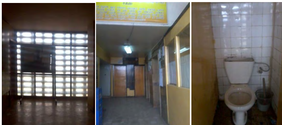
Figure 3- 70 Windows of the interior space and unventilated toilet
