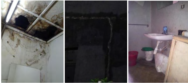
Figure 5- 3 Showing some of the problems in existing buildings caused by dampness and microbial growth
