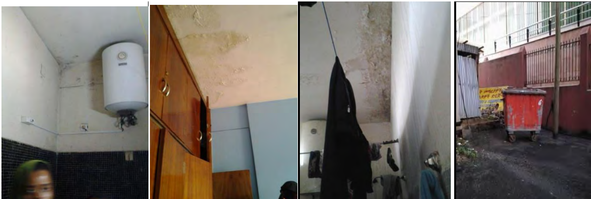
Figure 3- 32 Dampness caused by leakage and dampening of garbage near the play area
