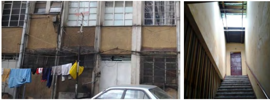
Figure 3- 15 Unpleasant looking façade because of leakage and dampness and effects of dampness due to open roof (from left to right)
