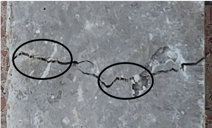
Figure 4.15. Bamboo fiber bridge crack (Zoomed)
