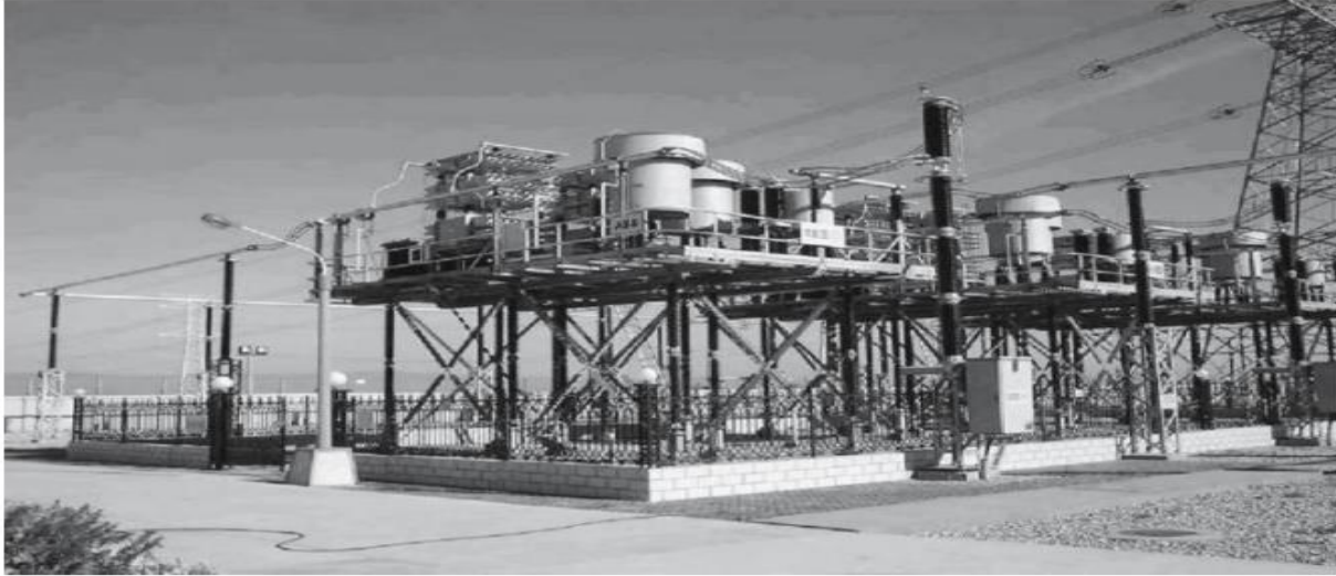
Figure 2.14 Series Compensation (Series Capacitor) (Source: ABB) [19]
