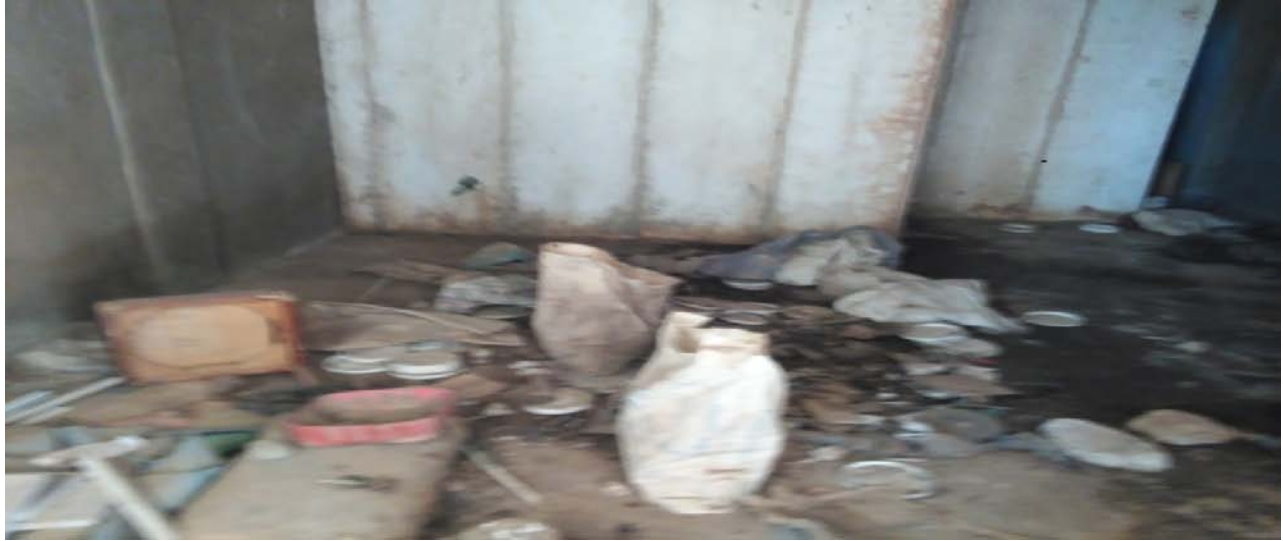
Photo1. The malfunctioning of the sewerage system in the condominiums, source: author
