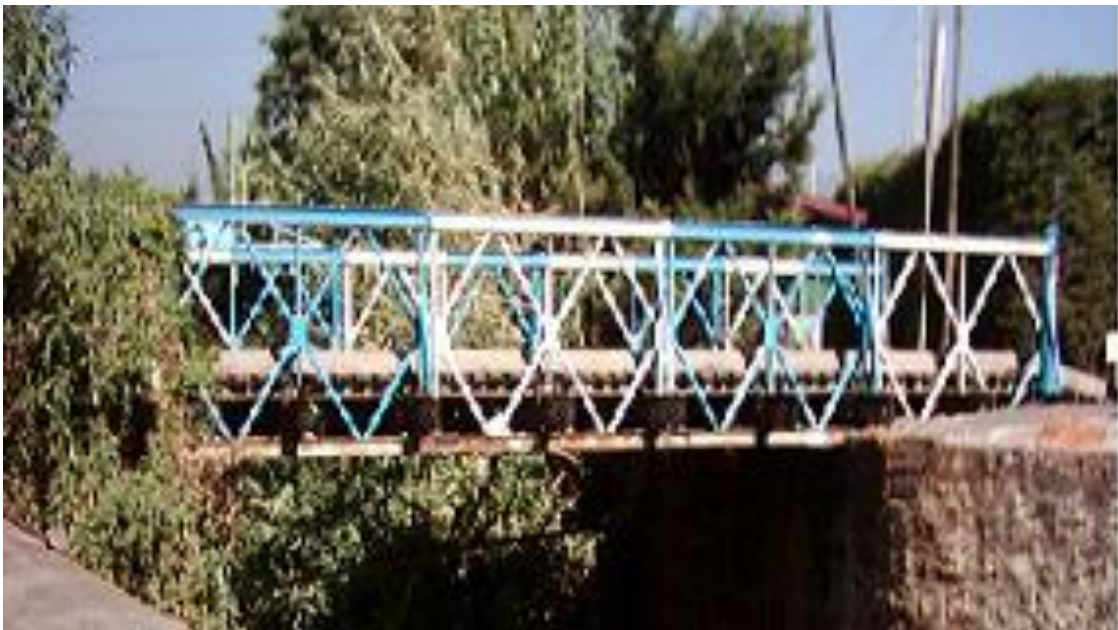
Figure 2.4: Baily truss bridge at the entrance to the Addis Ababa Tennis Club
