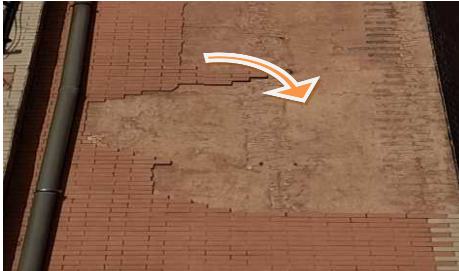
Figure 8 Picture of defect on external wall cladding
