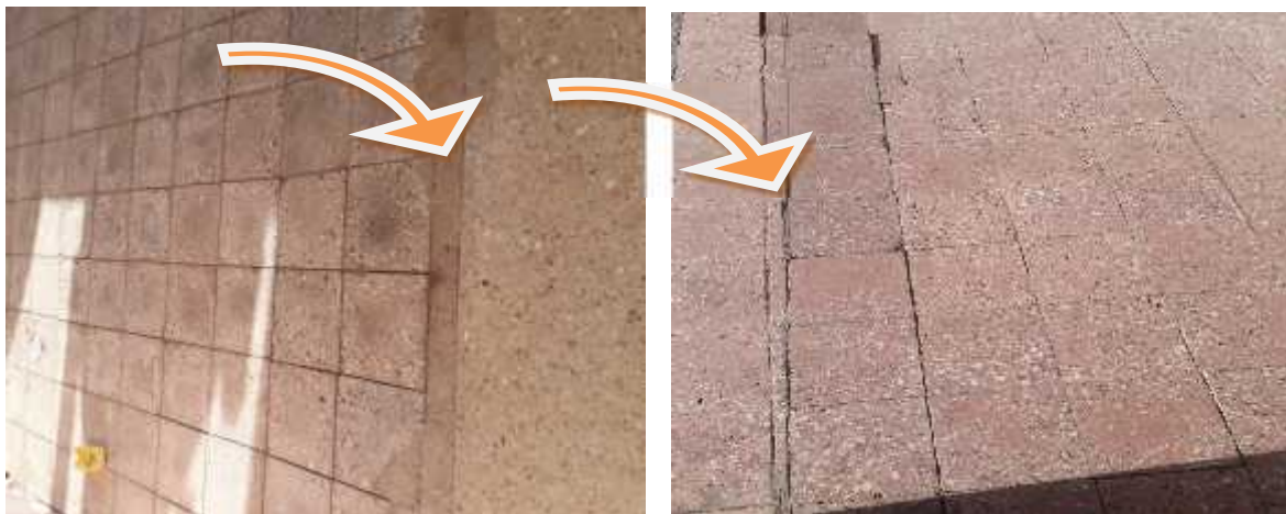
a) Poor connection method at ramp and floor b) Crack at grade beam and floor joint place
