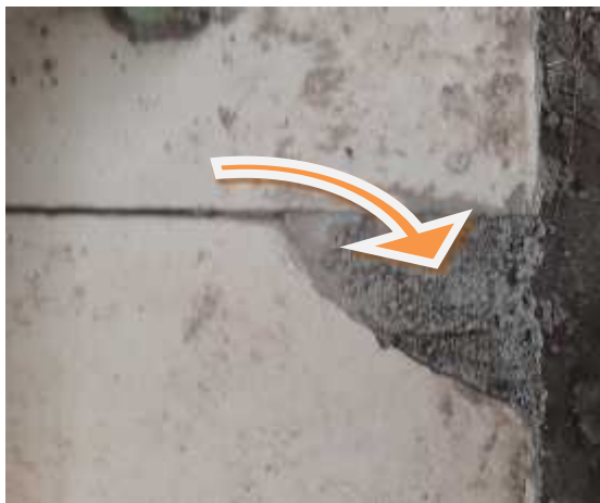
a) Broken ceramic floor tile
