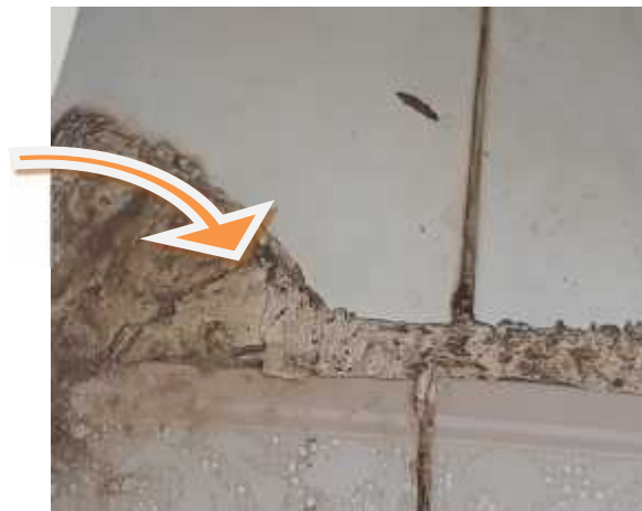
b) Broken ceramic floor tile
