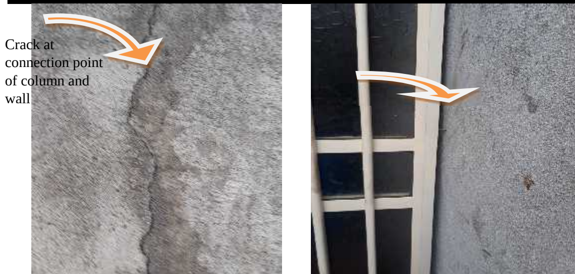
a) Crack at joint b/n column and HCB wall b) vertical wall plumping problem
