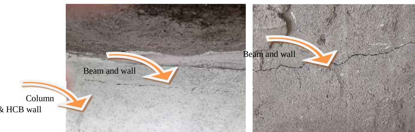
c) Crack at joint between beam and HCB wall d) Crack at joint between beam and wall and column and hollow concrete block wall
