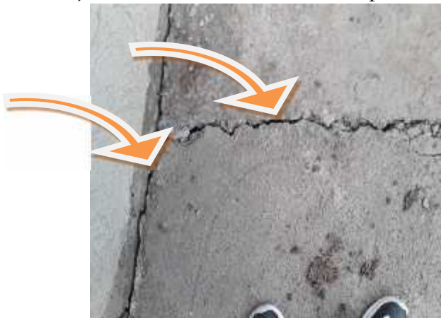
c) Cracked on pavement around building
