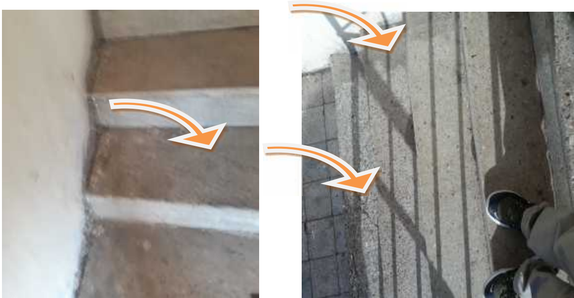
c)Unclean tread& mortar mixed on it, d) Cracked tread and short length
