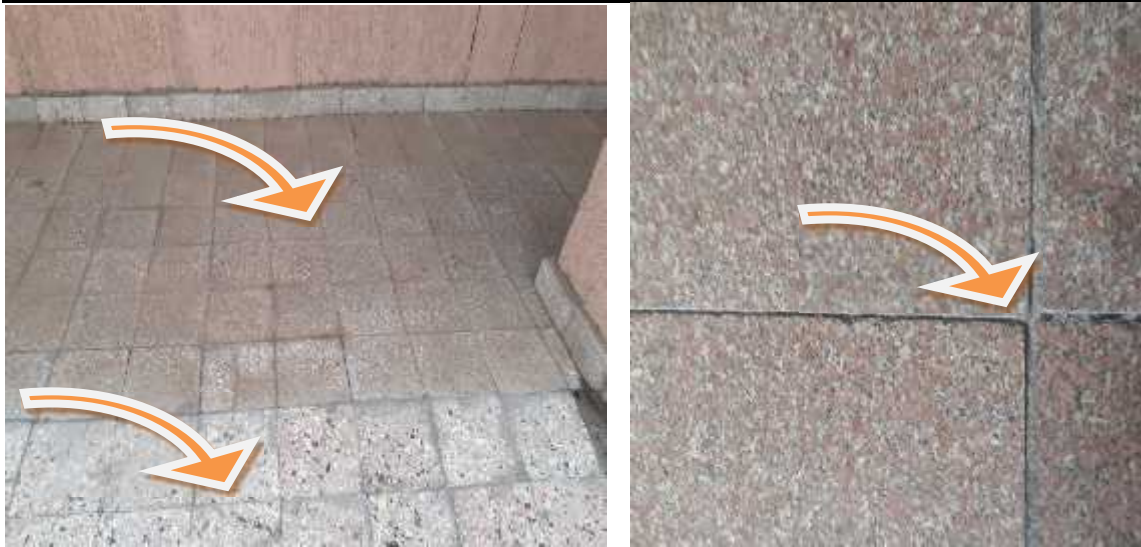
e) Different type of terrazzo tile and level problem f) Alignment and grouting defect
