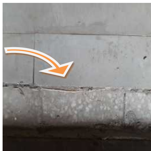
b) Poor workmanship at marble and terrazzo floor joint
