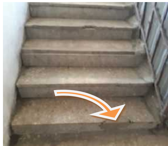
b)Broken tread has been rectified by mortar
