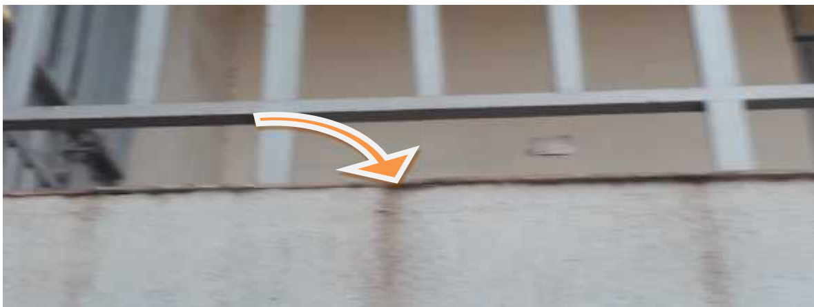
Figure 7 Picture of defect on balcony external wall.
