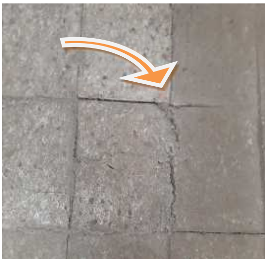
a) Damaged terrazzo tile
