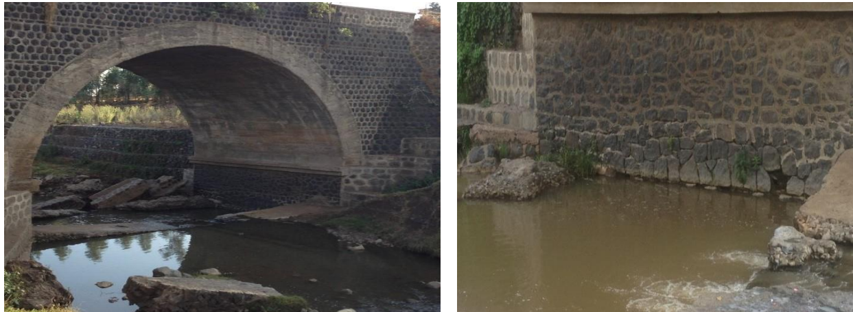
Figure 1-1: Bridge scour problem at the River bed and Abutment of Ginchi Awash Bridge (April 02, 2018).
