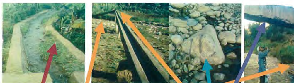
Figure 14. Condition of the lined canals and flume on the left side canals
