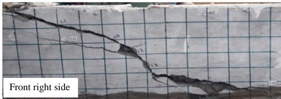
Figure 5-26 Just before failure cracks beam 75DCB2
