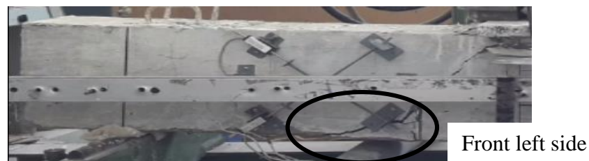
Figure 5-43 Beam 75BB1 critical diagonal crack
