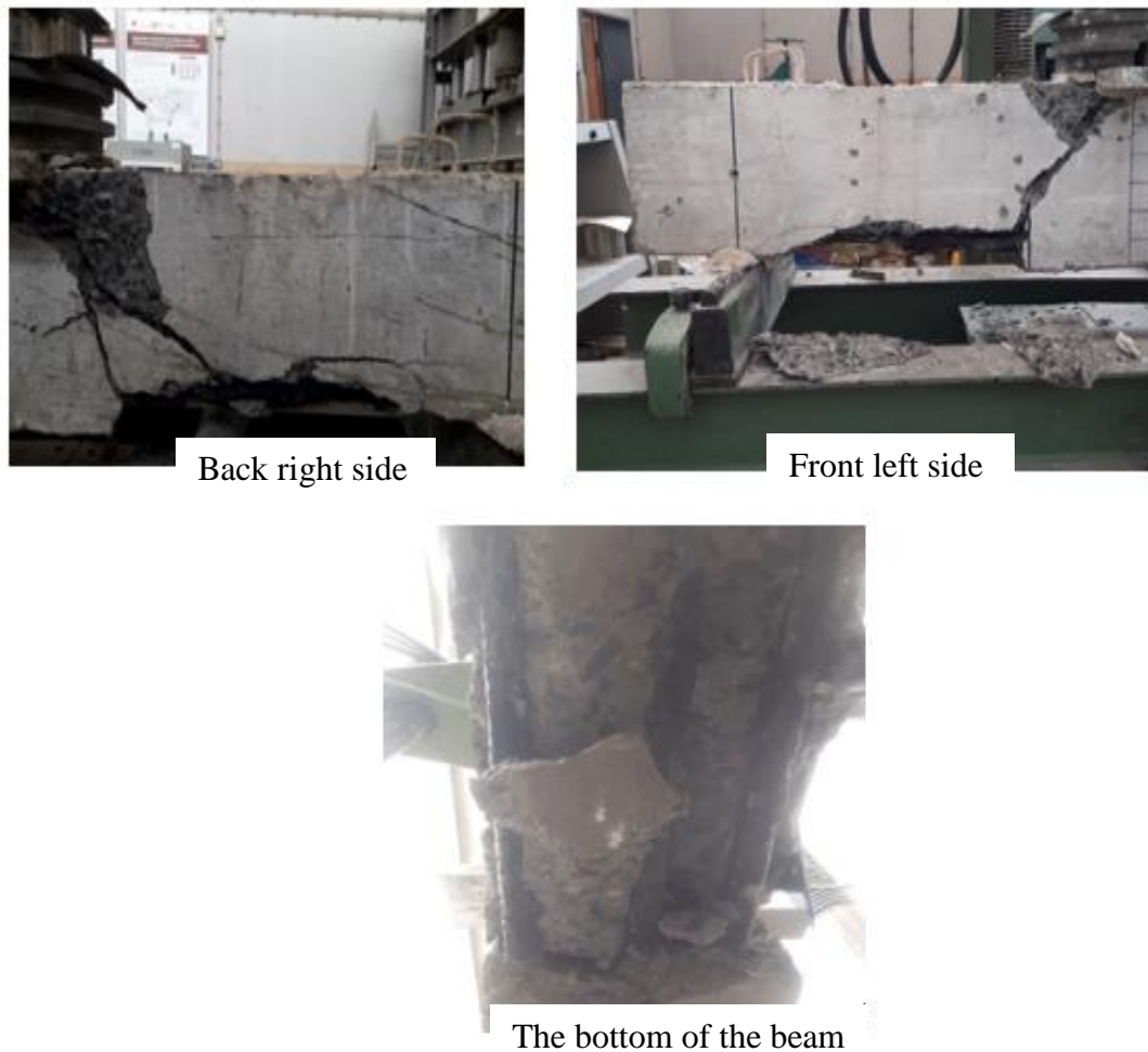
Figure 5-12 Close up on the cracks of beam 75BB2
