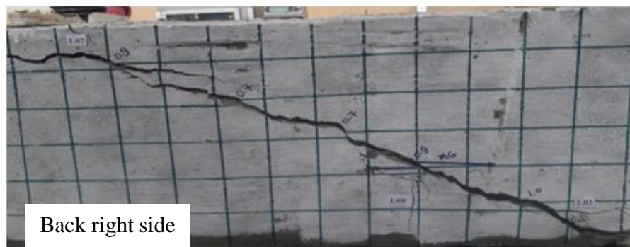
Figure 5-19 Close up on the cracks of beam 50DCB2
