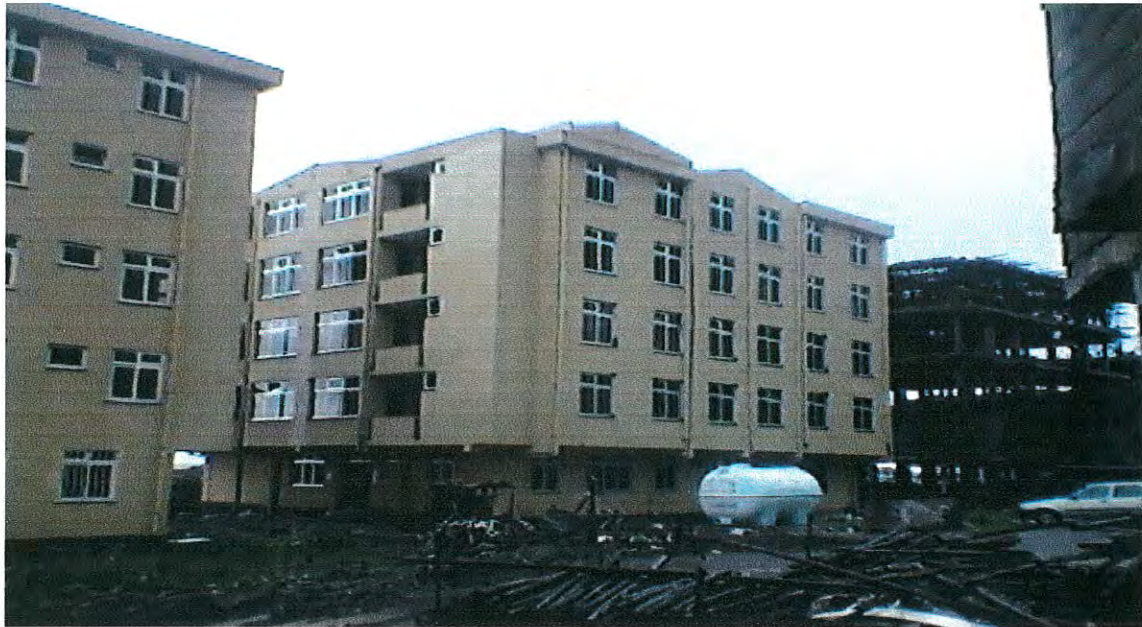
Figure 4.7: Apartments of Ayat Real Estate which are Under Construction at Ayat Site
