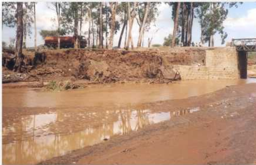
Figure 2.6: Eroded Embankment on Konso side of Dilbena river crossing.
