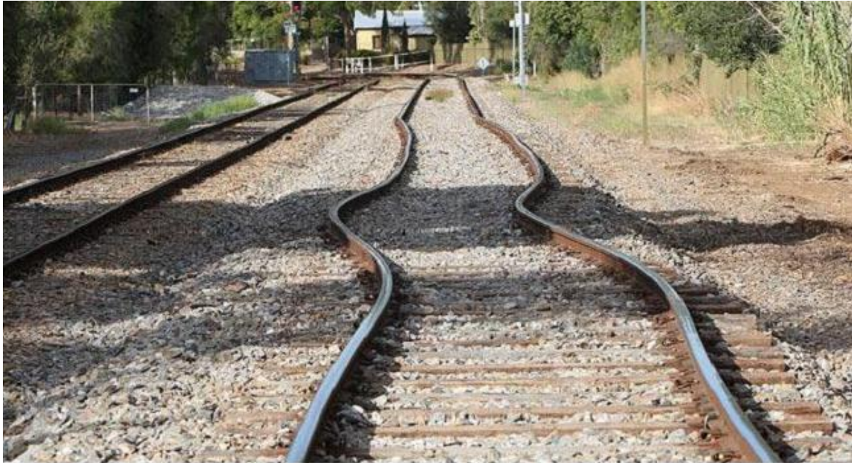
Figure 1-1:-Rail buckling (Telegraph Media Group, 2010)
