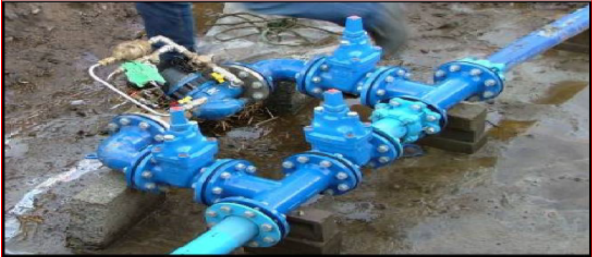
Figure 4 -3: Typical installation of P RV.
