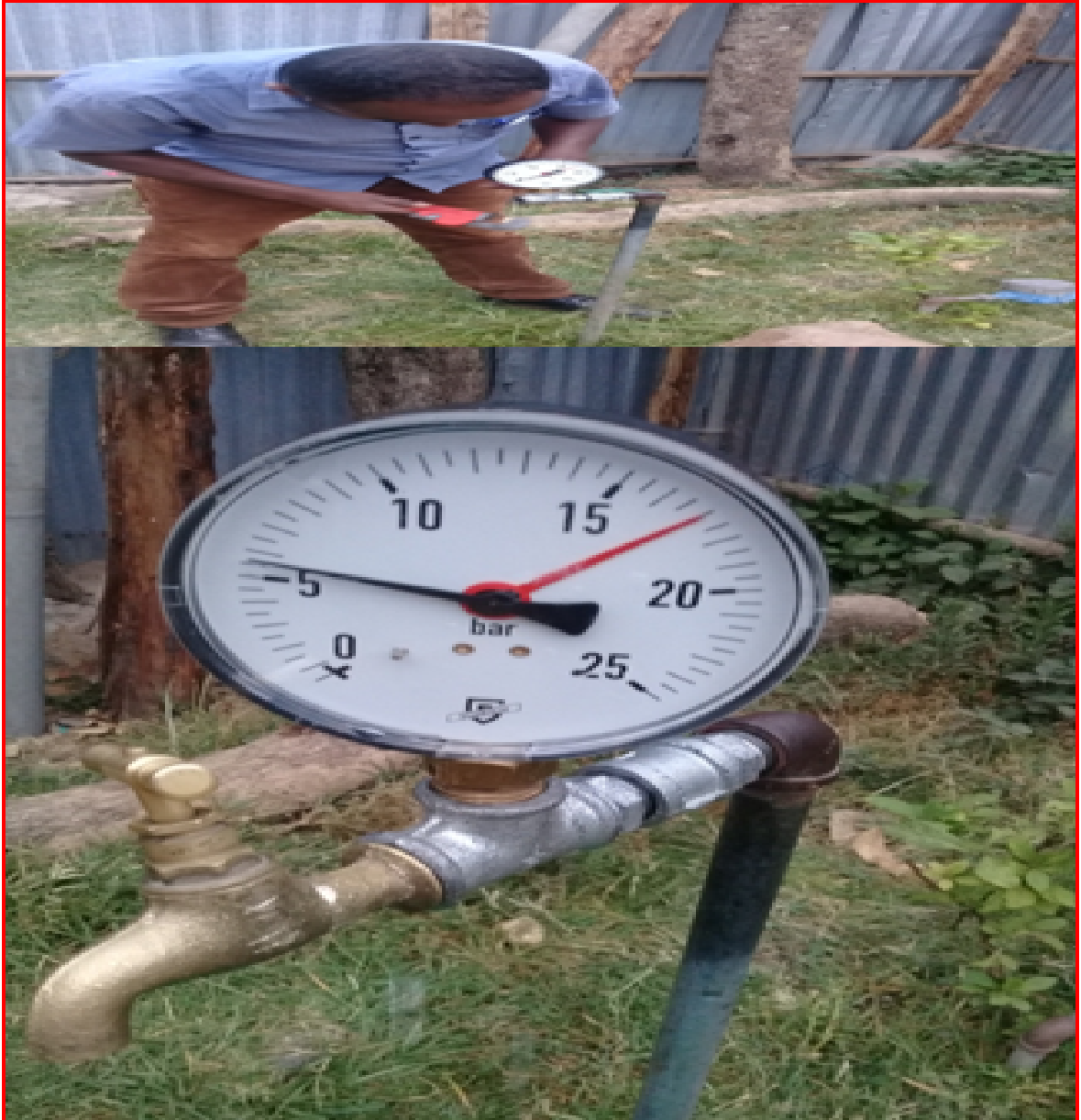
Figure 3-4: Shows Pressure measurement at faucet line at near of the main distribution line .
