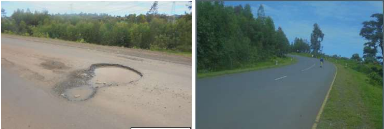
Figure: 4. 14 Road deterioration and vegetation coverage of Katta Fola
