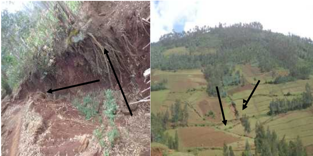
Figure: 5.2 Root exposures and gully
