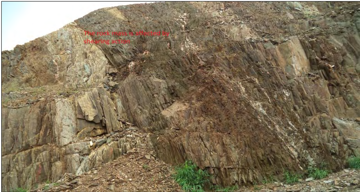
Plate 2.4: The rock mass found on top of left abutment key trench excavation area is affected by shear zone and weathering actions
