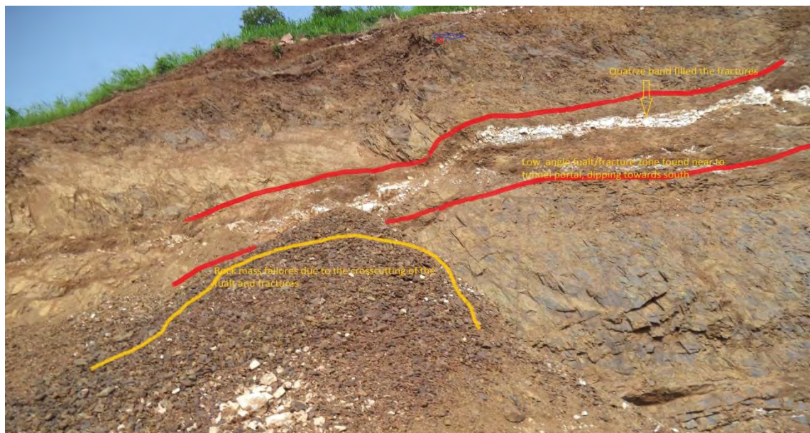
Plate 2.5: Low angle fault/ fracture zones encountered at the outlet tunnel portal area, dipping 20^{\circ} to 25^{\circ} towards south east.
