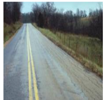
Figure 2-2: Picture of Edge Crack
