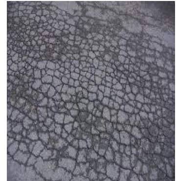
Figure 2-1: Picture of Alligator Crack
