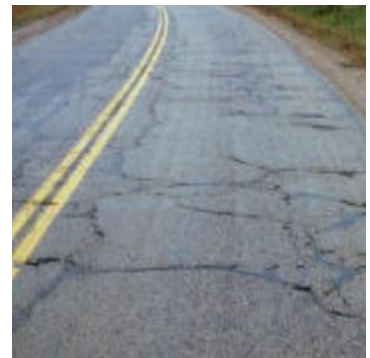
Figure 2-3: Picture of Block Crack
