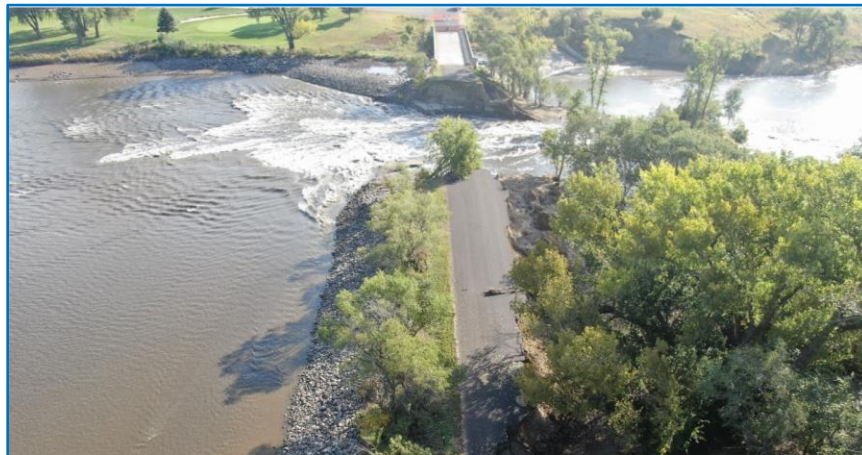
Figure 2. 2: Platte Dam Breached Drone Footage (ASDSO, 2020)
