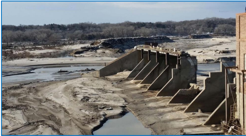
Figure 2. 3: Spencer Dam Breached Photo (ASDSO, 2020)
