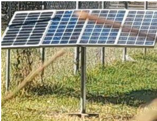
Figure 4. 9. Photovoltaic (PV) modules and 12- volt DC axial fan.
