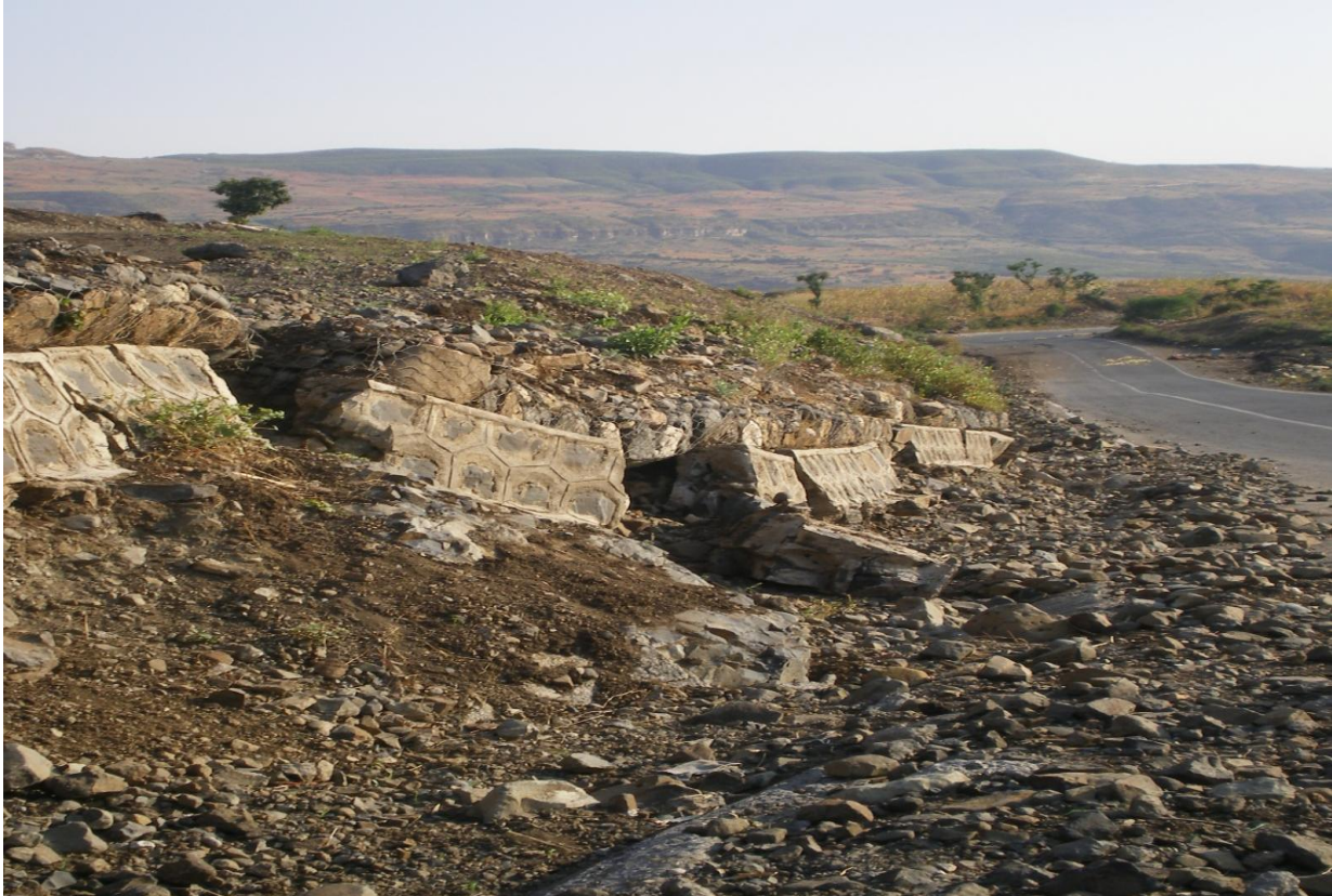
a) Falling masonry retaining wall
