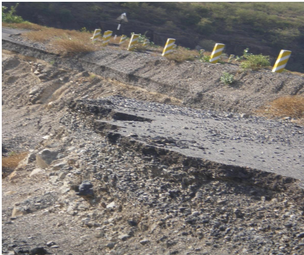
Figure 1-8 View of the land slide at ST-22
