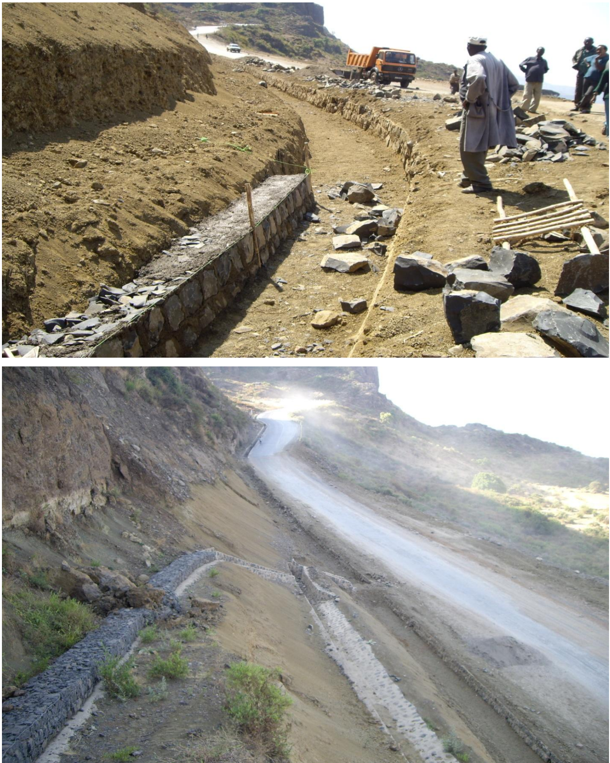
Figure 1-4 View of the land slide at ST-1
