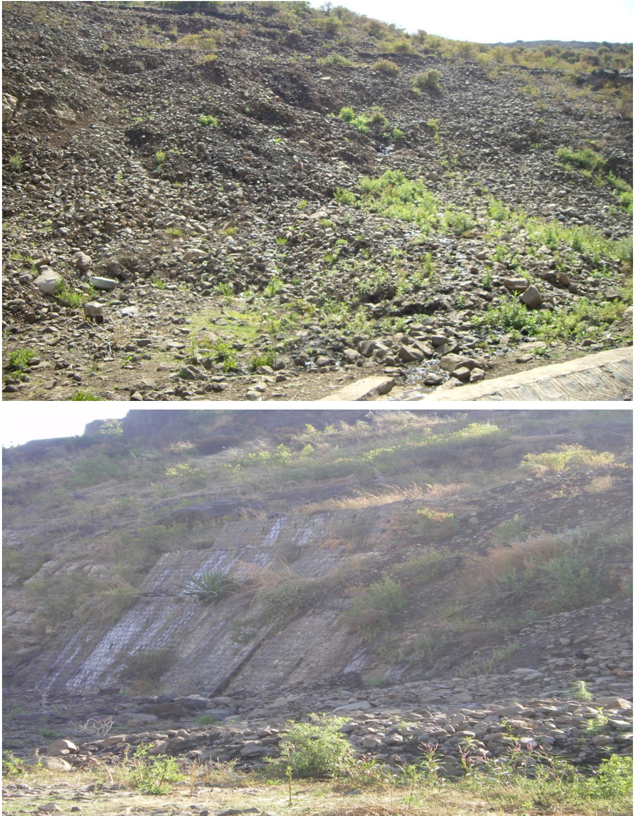
Figure 1-6 View of the land slide at ST-05
