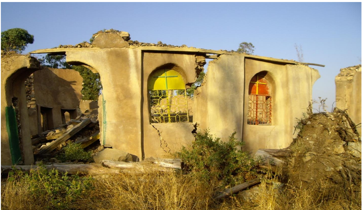
b) Collapsed church
