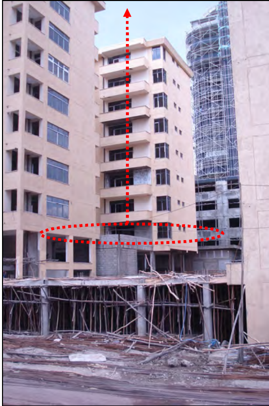
Pic - 3.4: Building height and massing problems.
