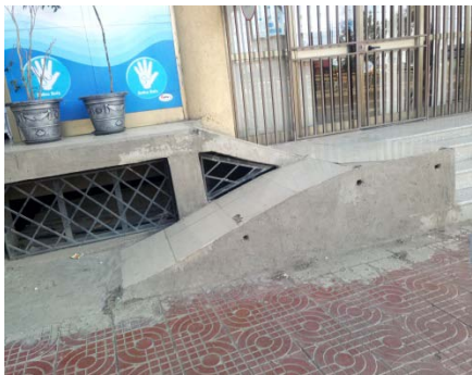
Ramps that have no handrail, too sloppy and slippery surface
