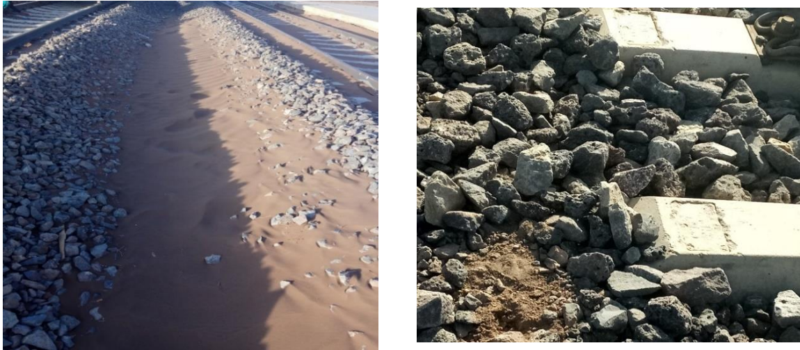
Figure 3-3 Ballast fouling condition on the line
