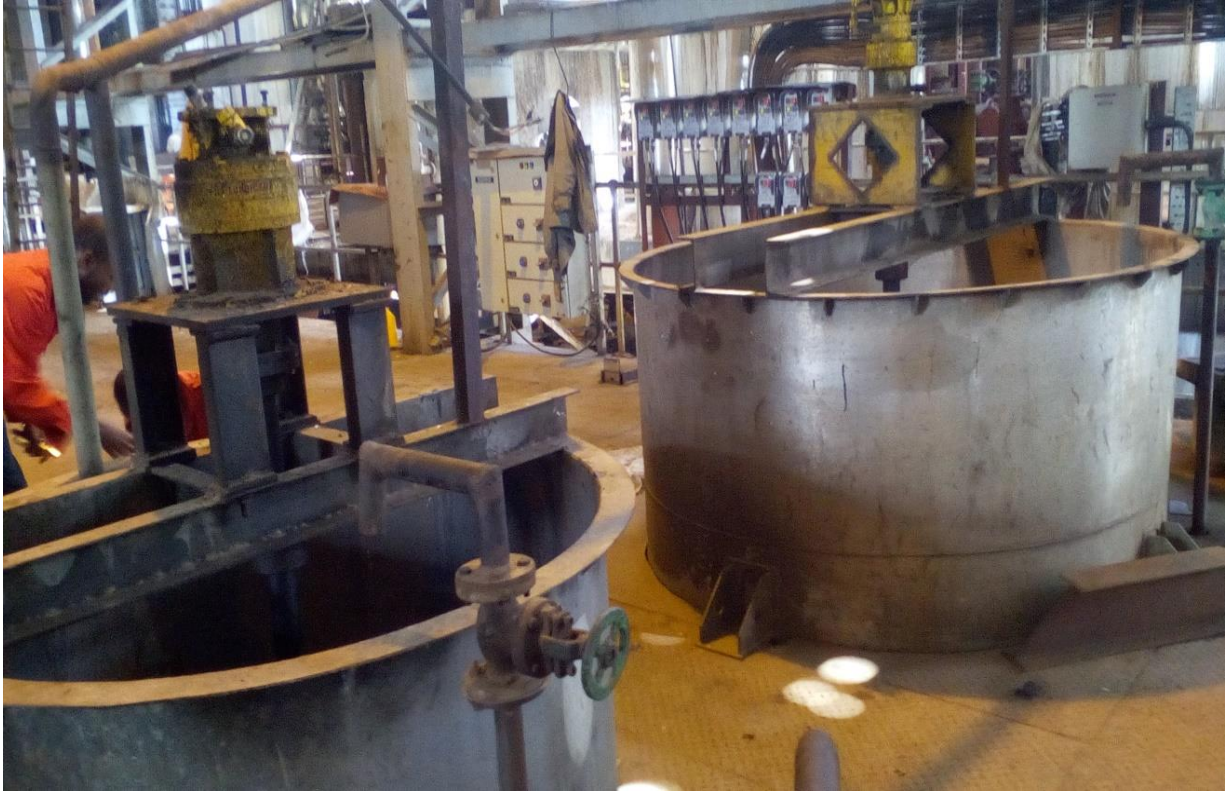
Appendix Photo 3. Flotation system syrup clarification plant
