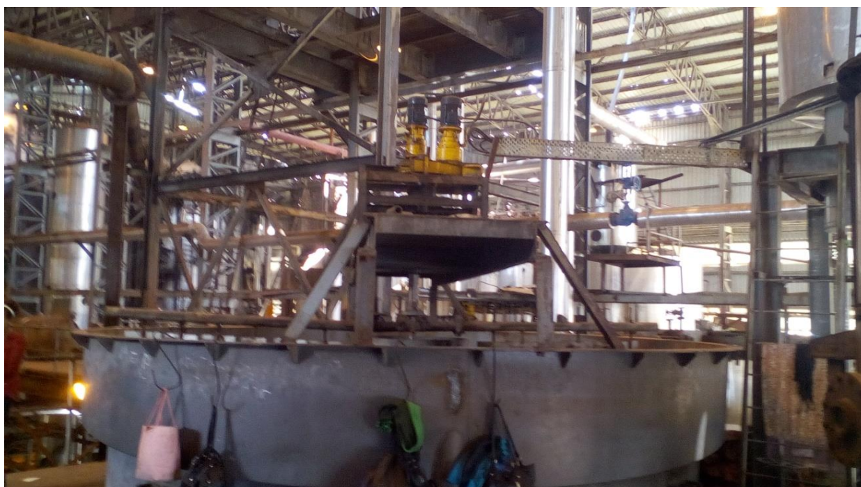
Appendix Photo 2. Flotation system syrup clarification plant
