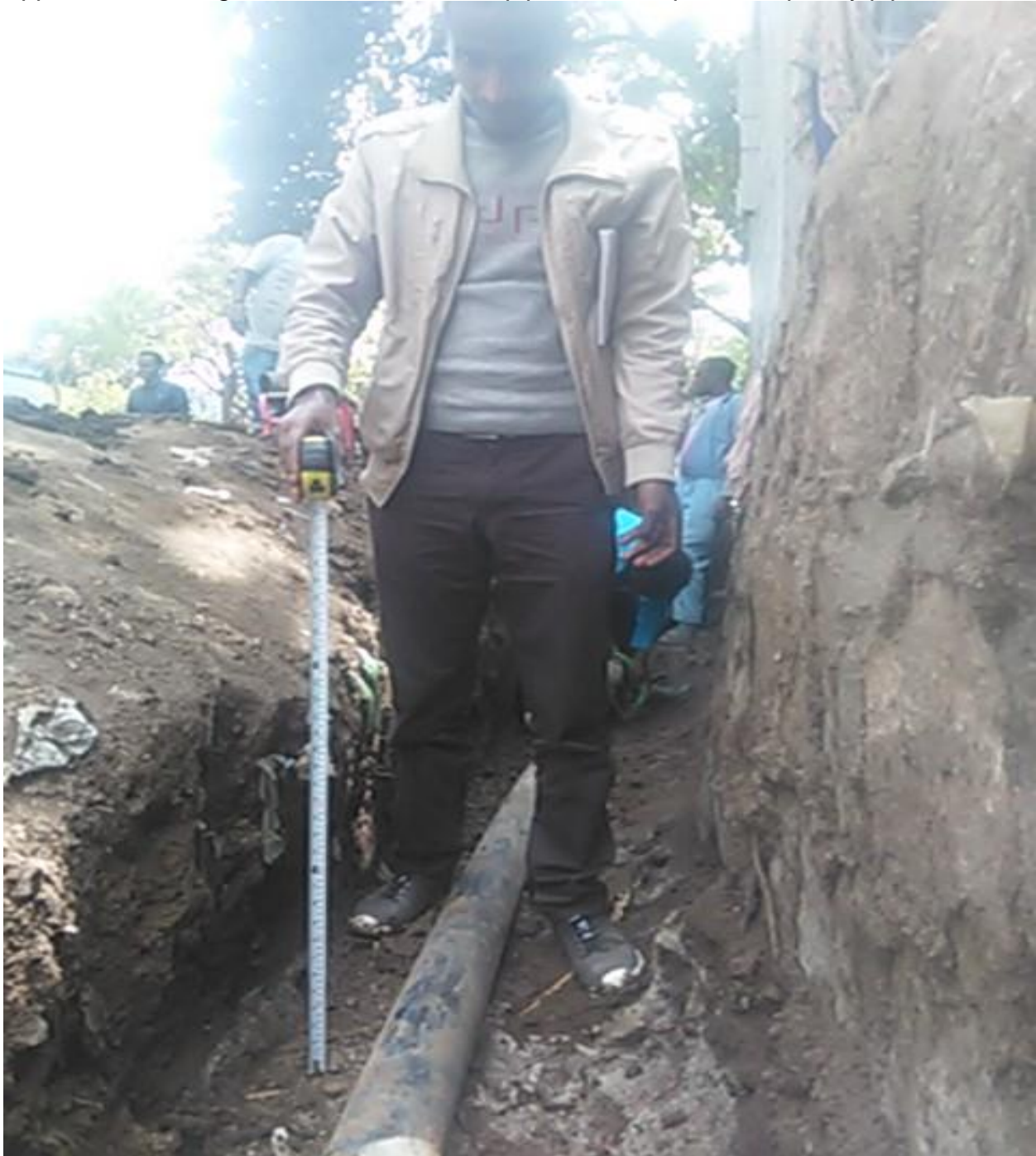
Appendix E: During field measures of total pipe buried depth at frequently pipe burst
