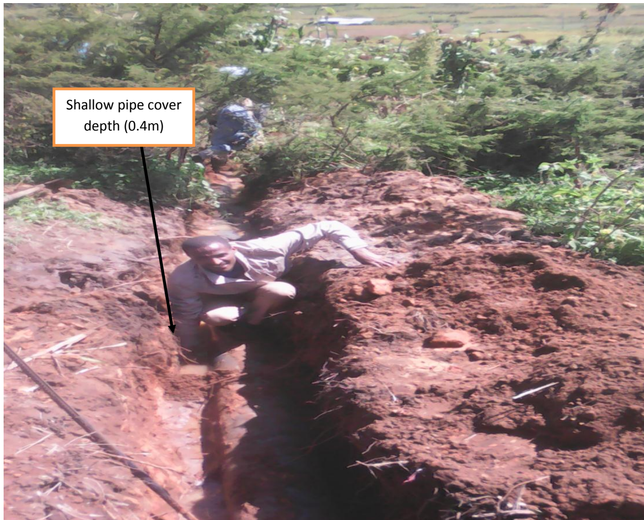
Figure 4.5.3 uPVC pipe burst insufficient buried depth
