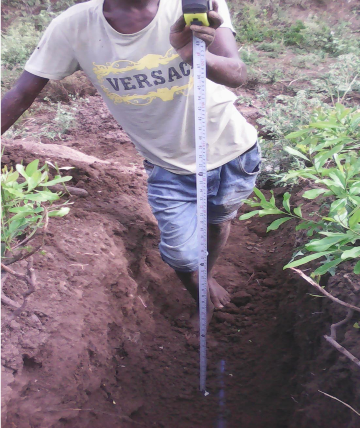
Appendix F: During field measures of total pipe buried depth at no pipe burst appeared
