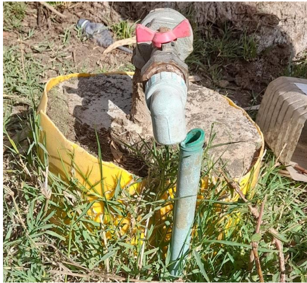
Figure 25. The picture of broken pipe when trying to maintained the stacked valve
